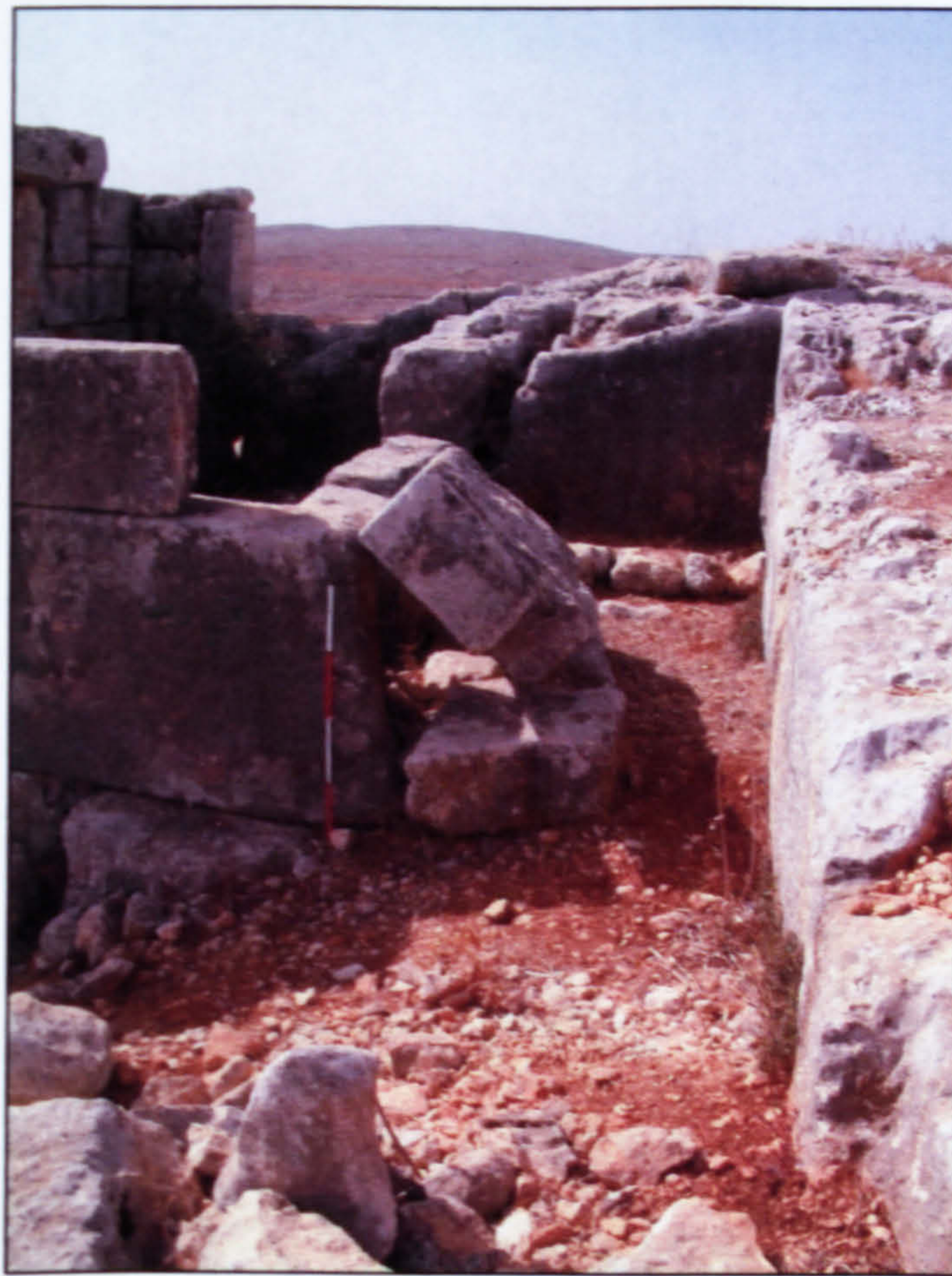
Figure 111: Access to the second storey of the press building from the monastic site
