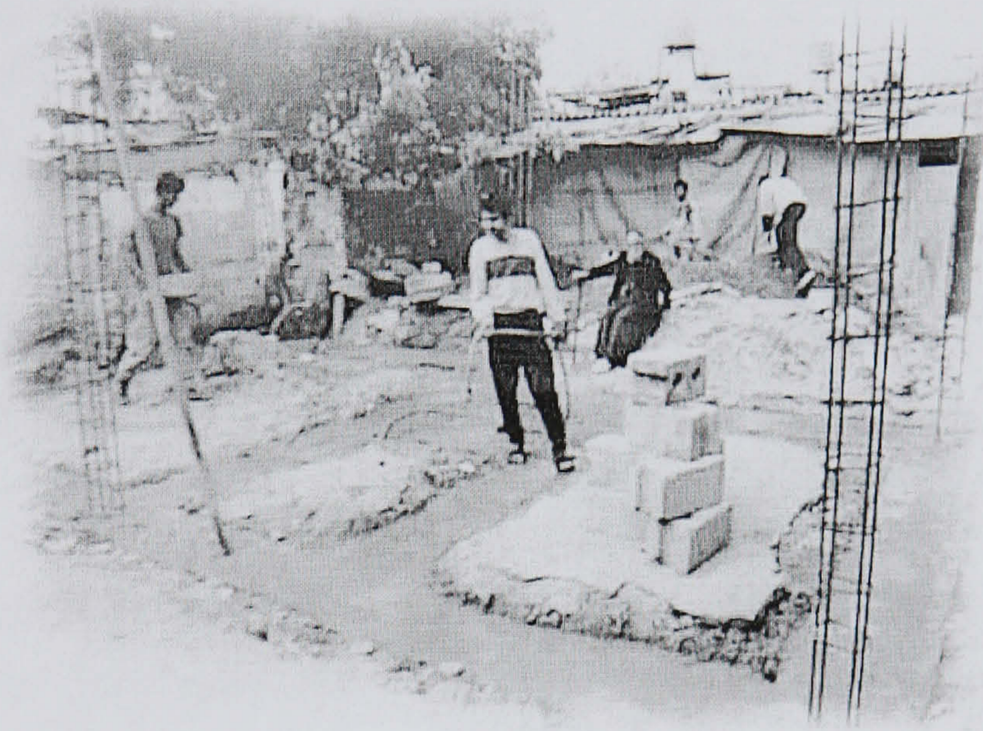
Figure 6.5: Shelter Rehabilitation Programme in One of the Refugee Camps. Source: The Courtesy of UNRWA.
