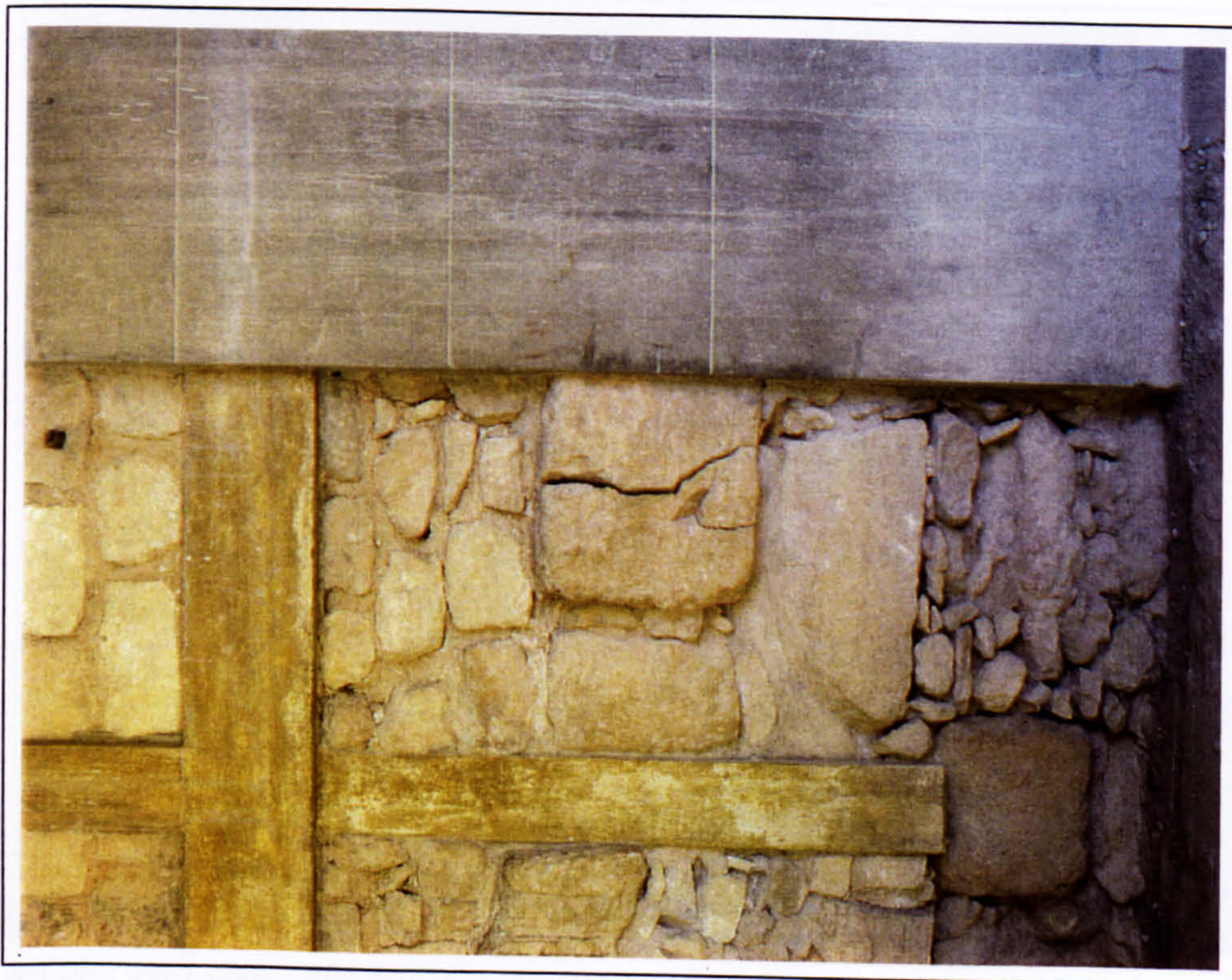
Plate 156 Hall of the Double Axes: crack of a stone which was partly incorporated in the reconstructed concrete pillar and in the wall.
