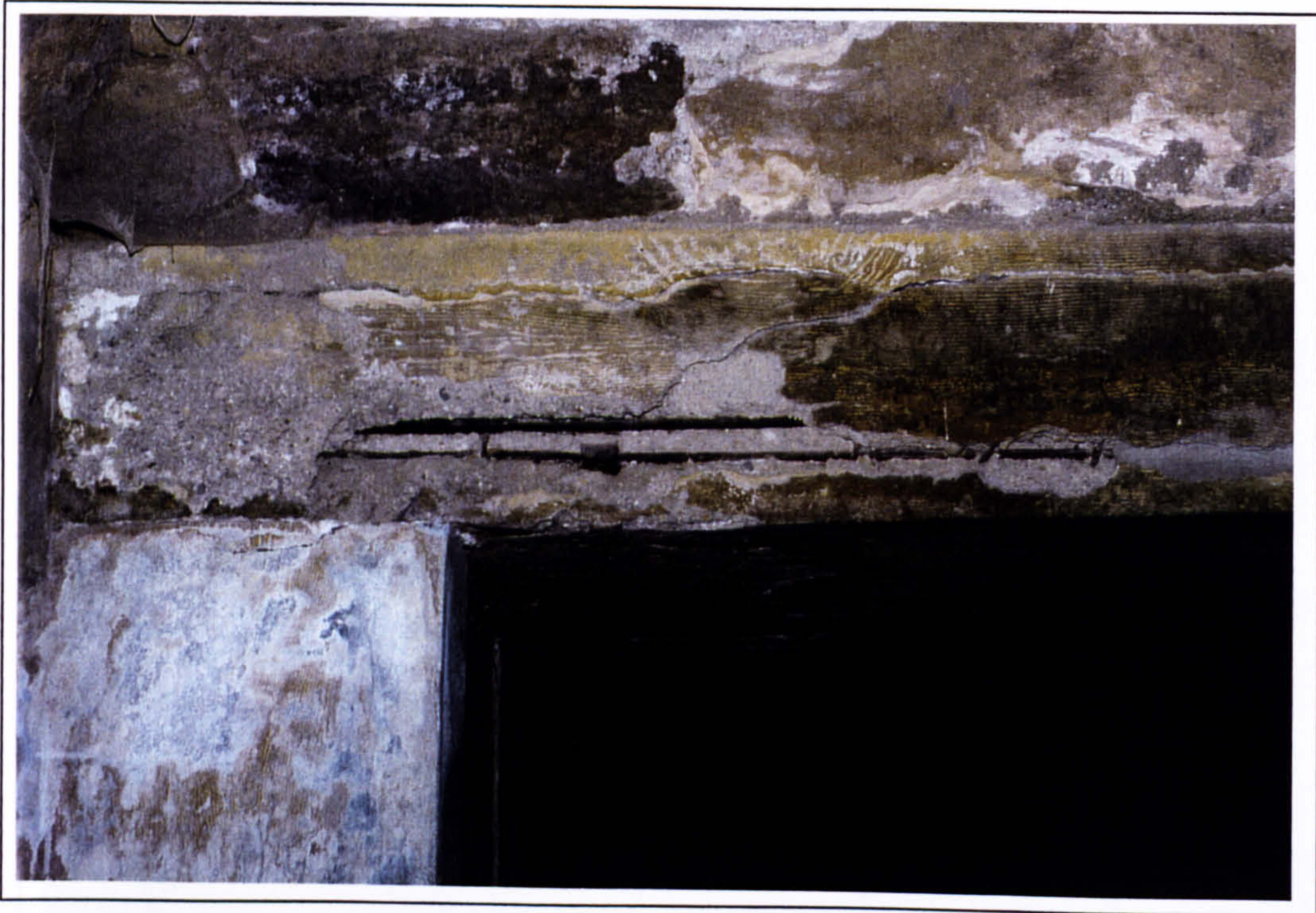
Plate 204 Door lintel in the Domestic quarter with rusting iron reinforcement exploding the concrete envelope. The lower line is the lower flange of Doll's I-beam the upper line is an additional round reinforcement bar by de Jong.
