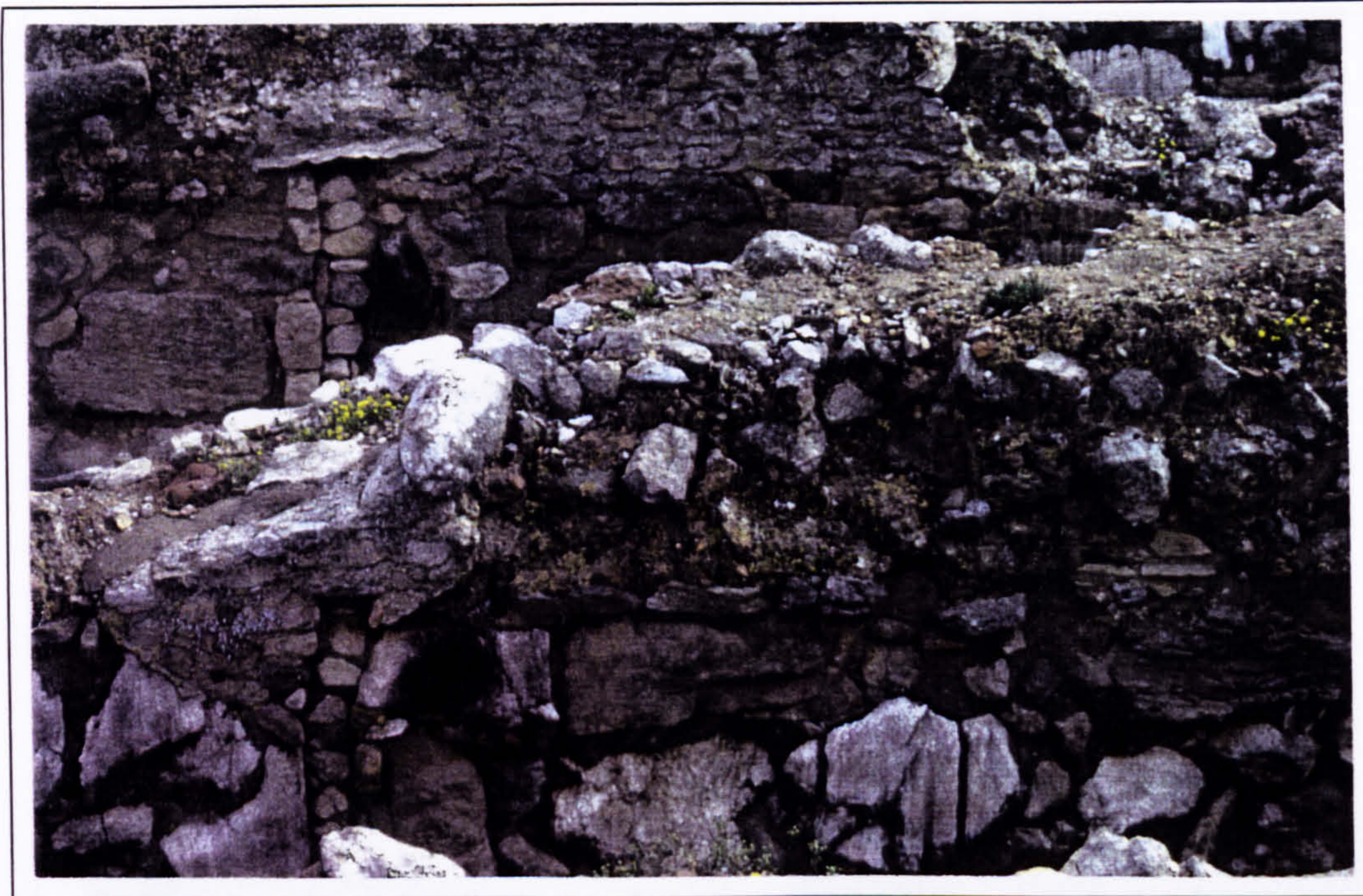
Plate 19 Walls of Magazine IV and V looking south, with rubble masonry infill in vertical slots. 1996.
