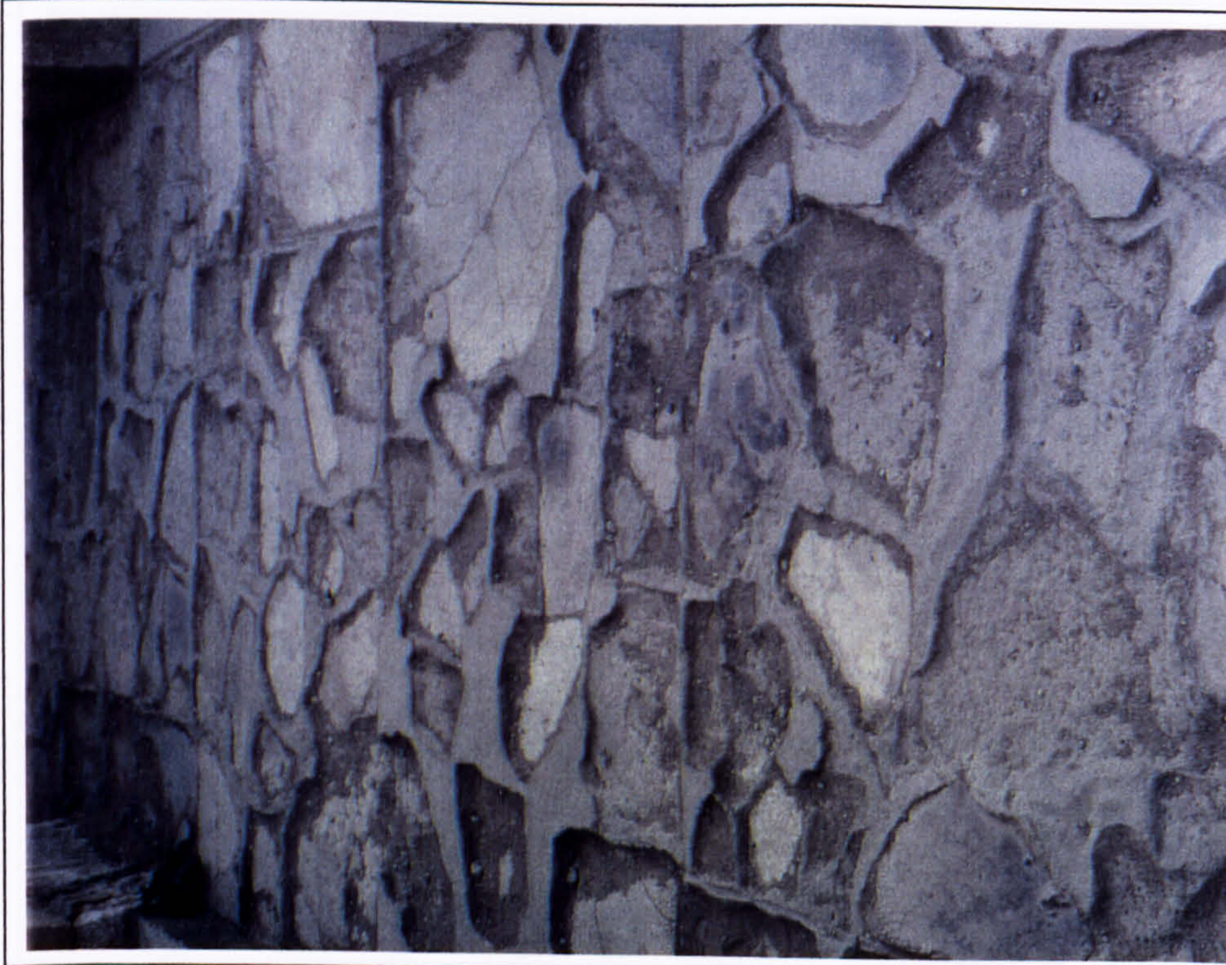
Plate 208 Decayed gypsum pavement in the upper East-West Corridor.
