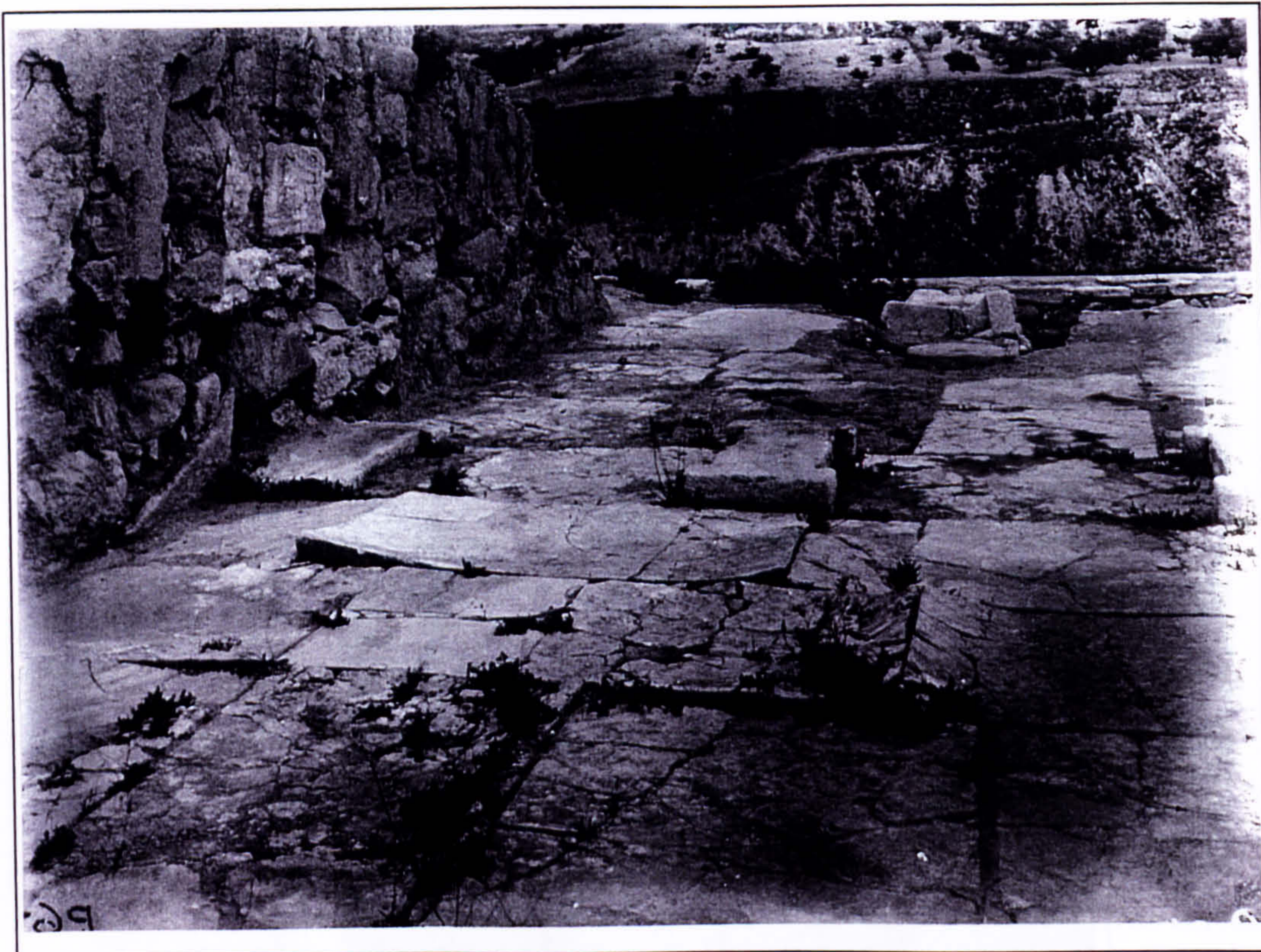
Plate 144 Decayed gypsum floor slabs in the Hall of the Double Axes. Date unknown, maybe 1910.
