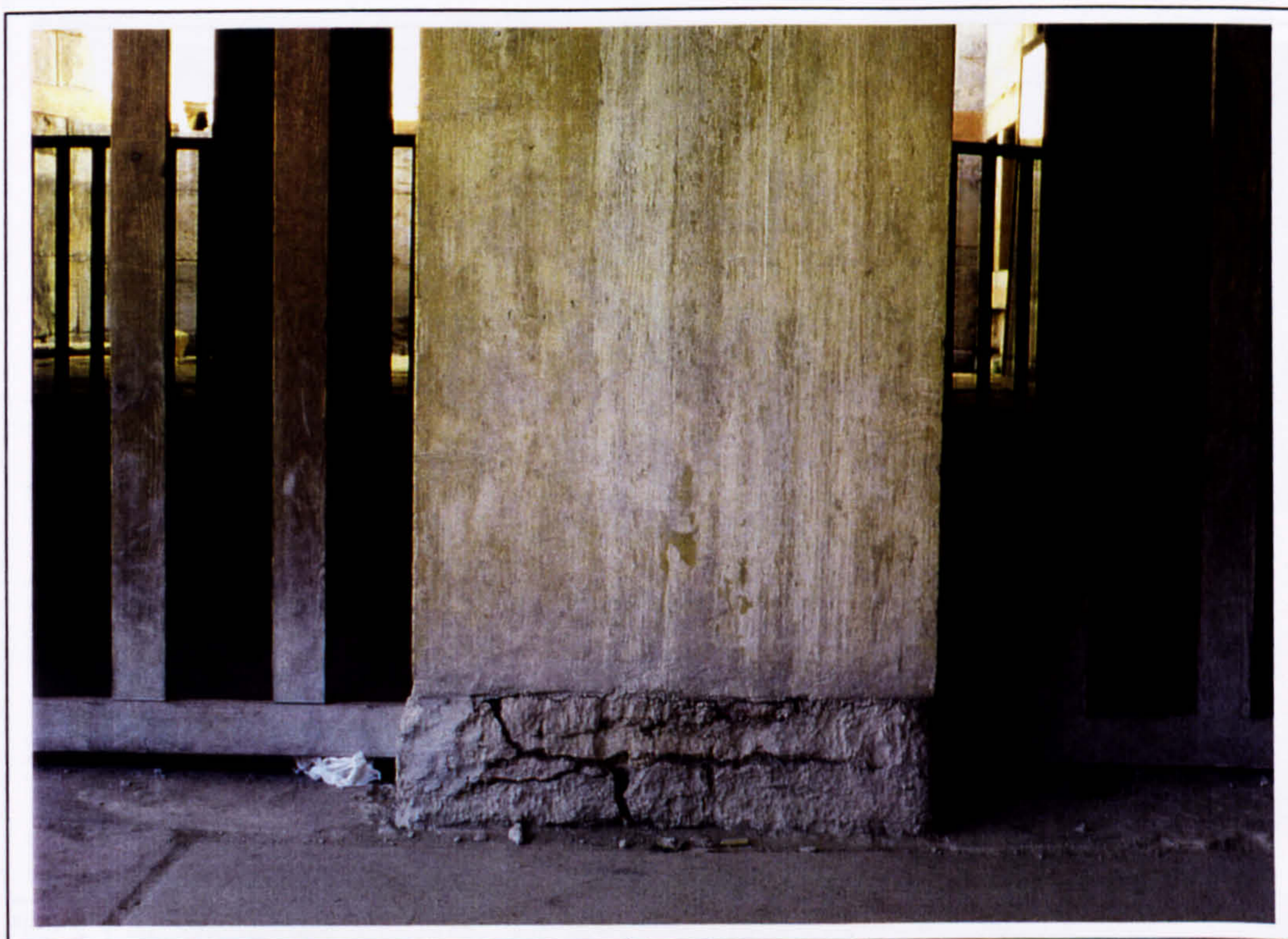
Plate 155 Original gypsum jamb block in the Hall of the Double Axes with superimposed new concrete Pillar in 1997.
