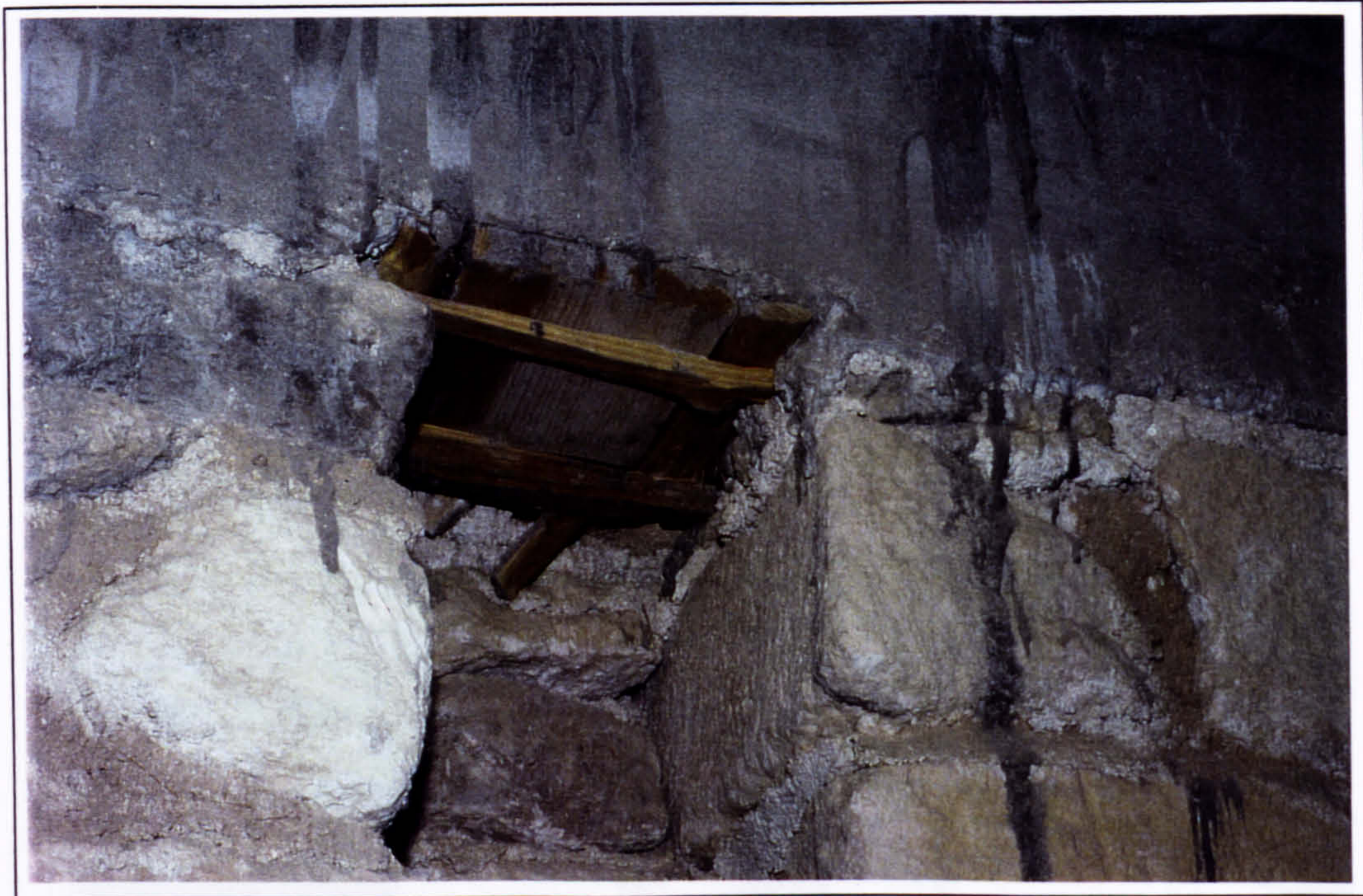
Plate 63 Shuttering of 1930 for concrete ring beam above slot in the Service wing in 1997.
