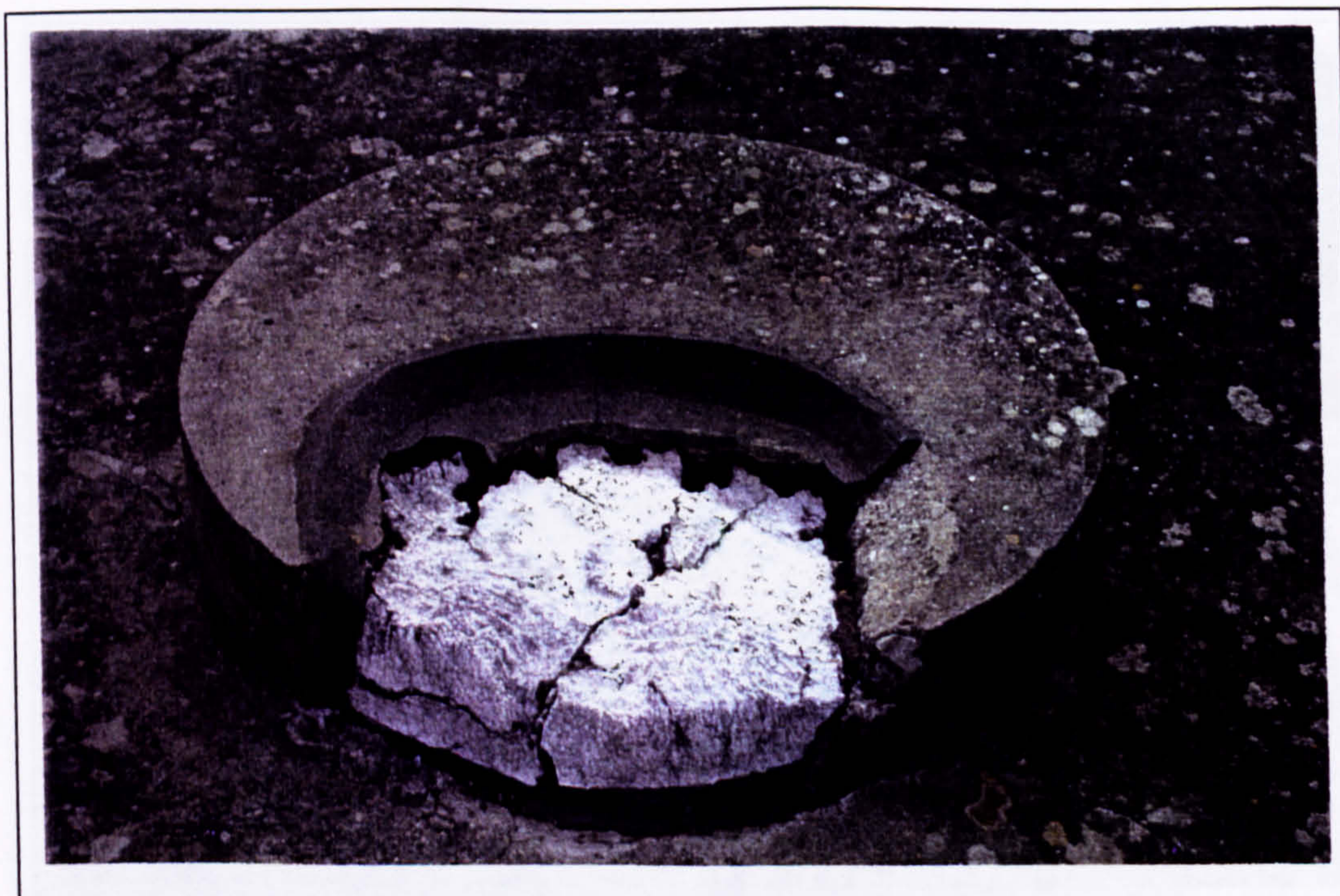
Plate 201 Remains of gypsum column base completed with concrete indicating supposed original height of the column base, the preserved level at the time of execution of the repair and the amount of weathering since then.
