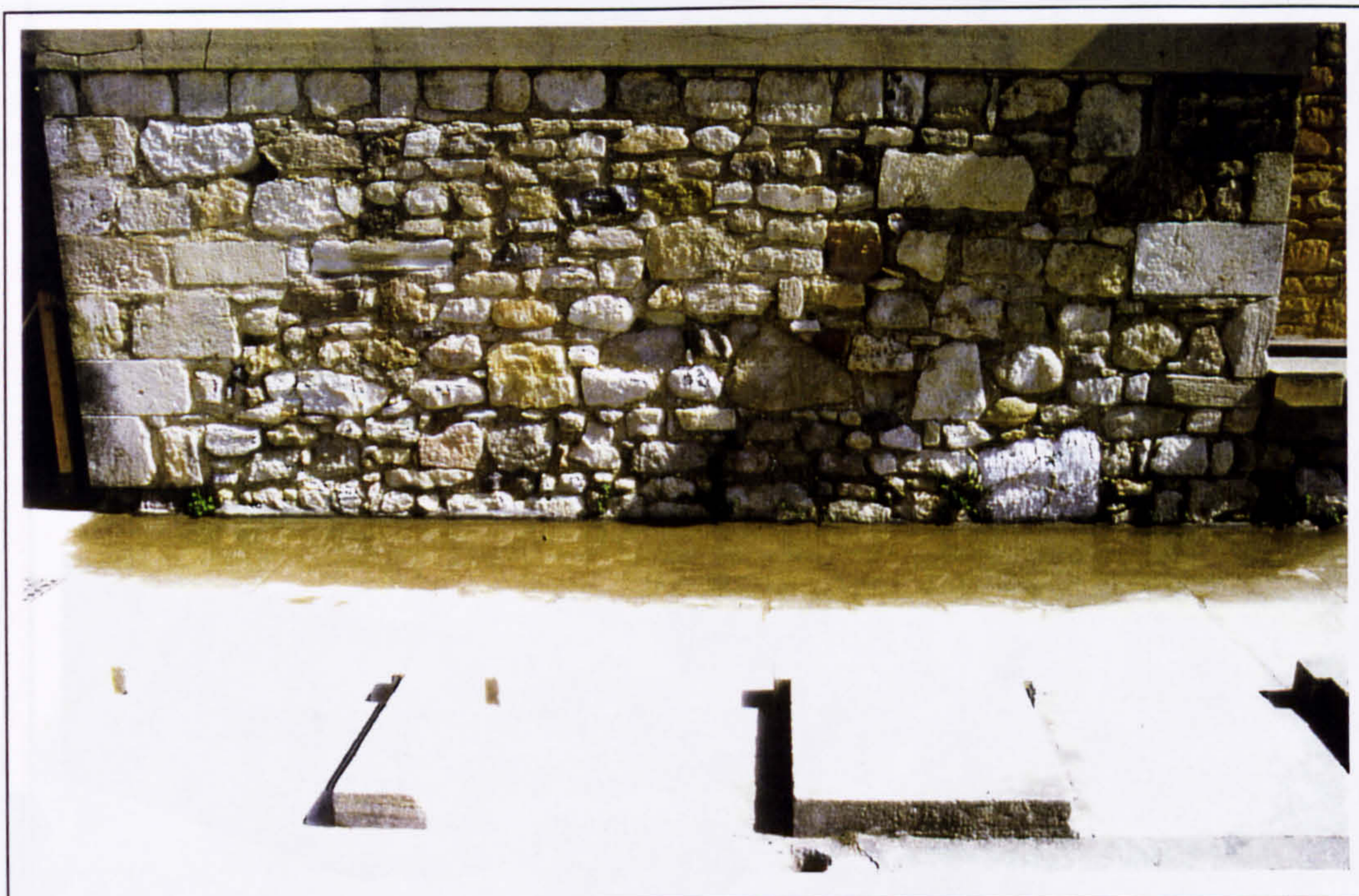
Plate 42 South face of the first floor middle wall of the Stepped Portico in 1997. Note the puddle indicating subsidence and the difference between the masonry of the 1922 reconstruction and of the 1923 work (one course below the concrete beam).
