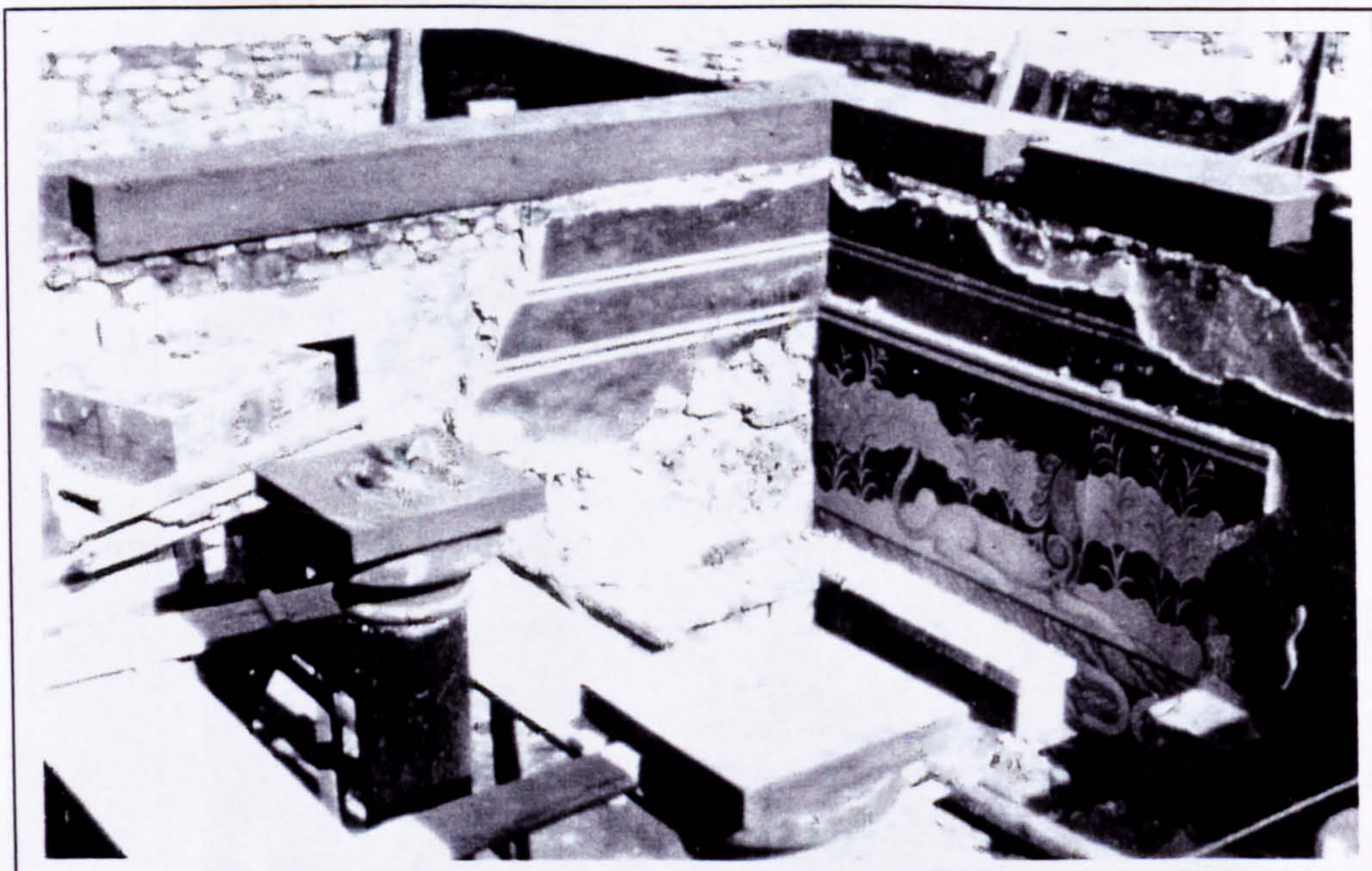
Plate 60 Construction of the concrete roof above the Throne Room in 1930. Note the ring beam with the mortices for ceiling beams.
