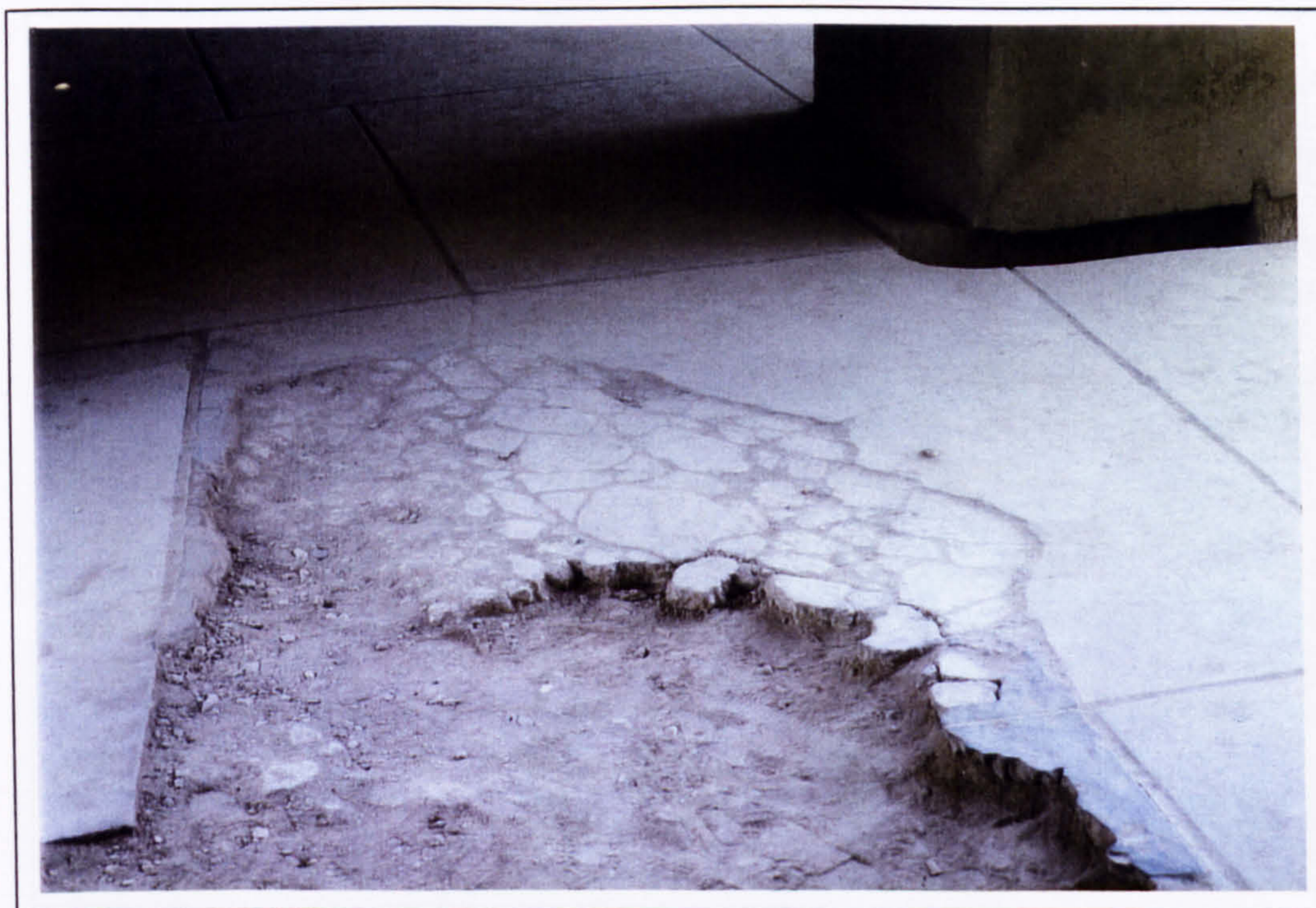
Plate 153 Decayed floor slab and concrete replacement slabs in the eastern portico of the Hall of the Double Axes in 1997.
