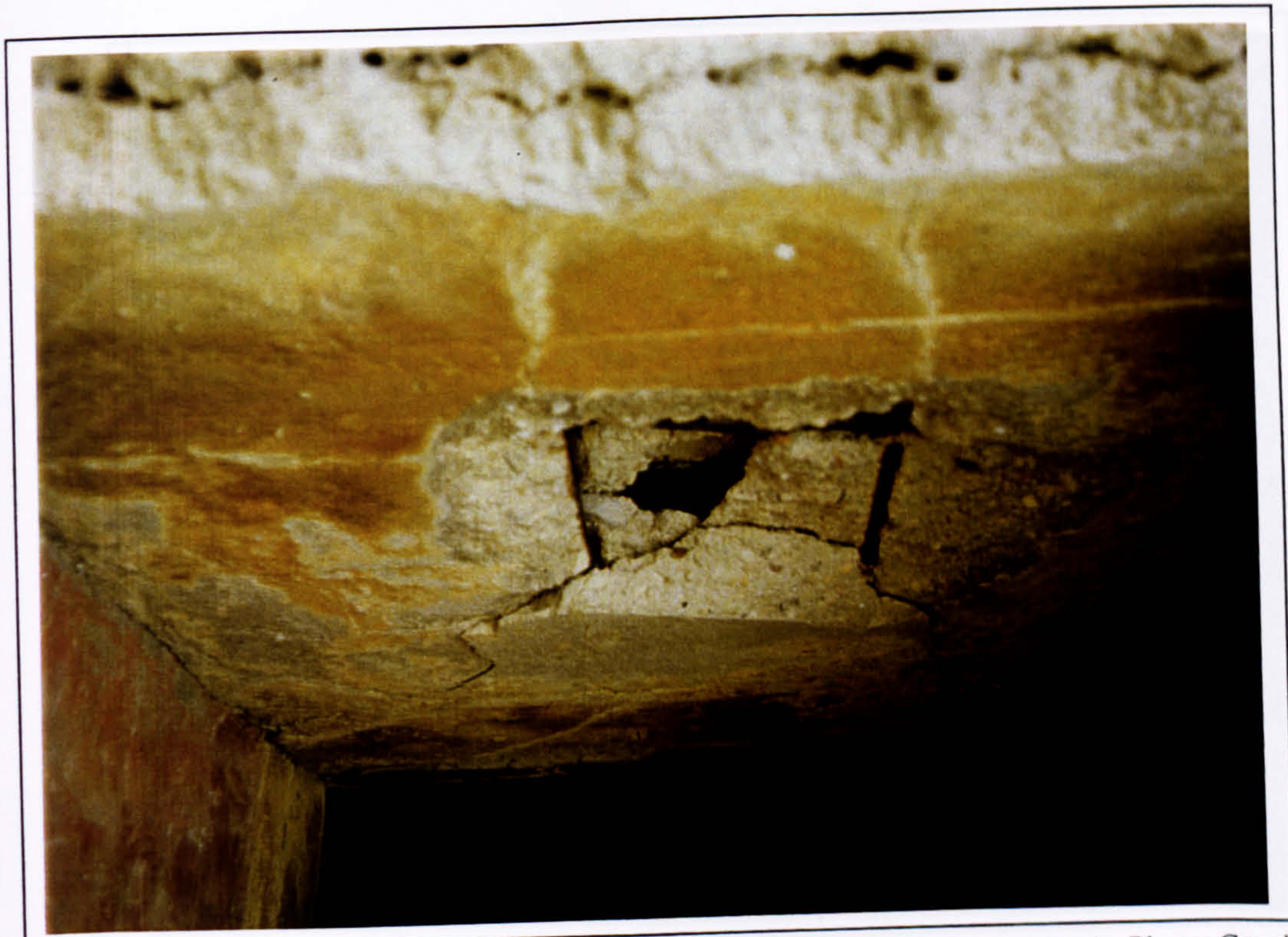
Plate 207 Lintel of the window between the Court of the Distaffs and the Room with the Plaster Couch with exposed iron-I-beam (centre) and reinforcement rods (left and right of centre).
