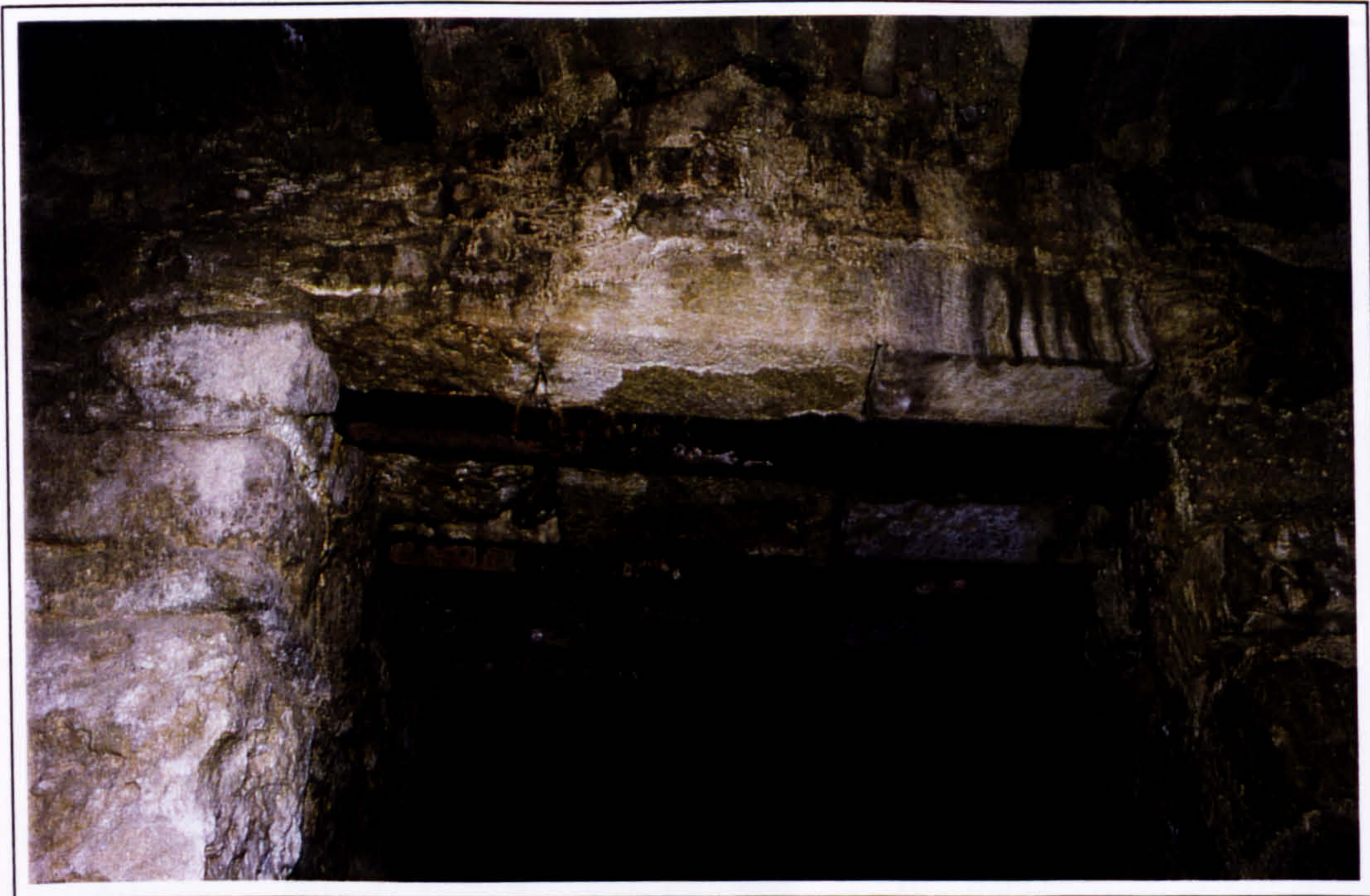
Plate 40 Lintel of the door between the two magazines beneath the Stepped Portico in 1997.
