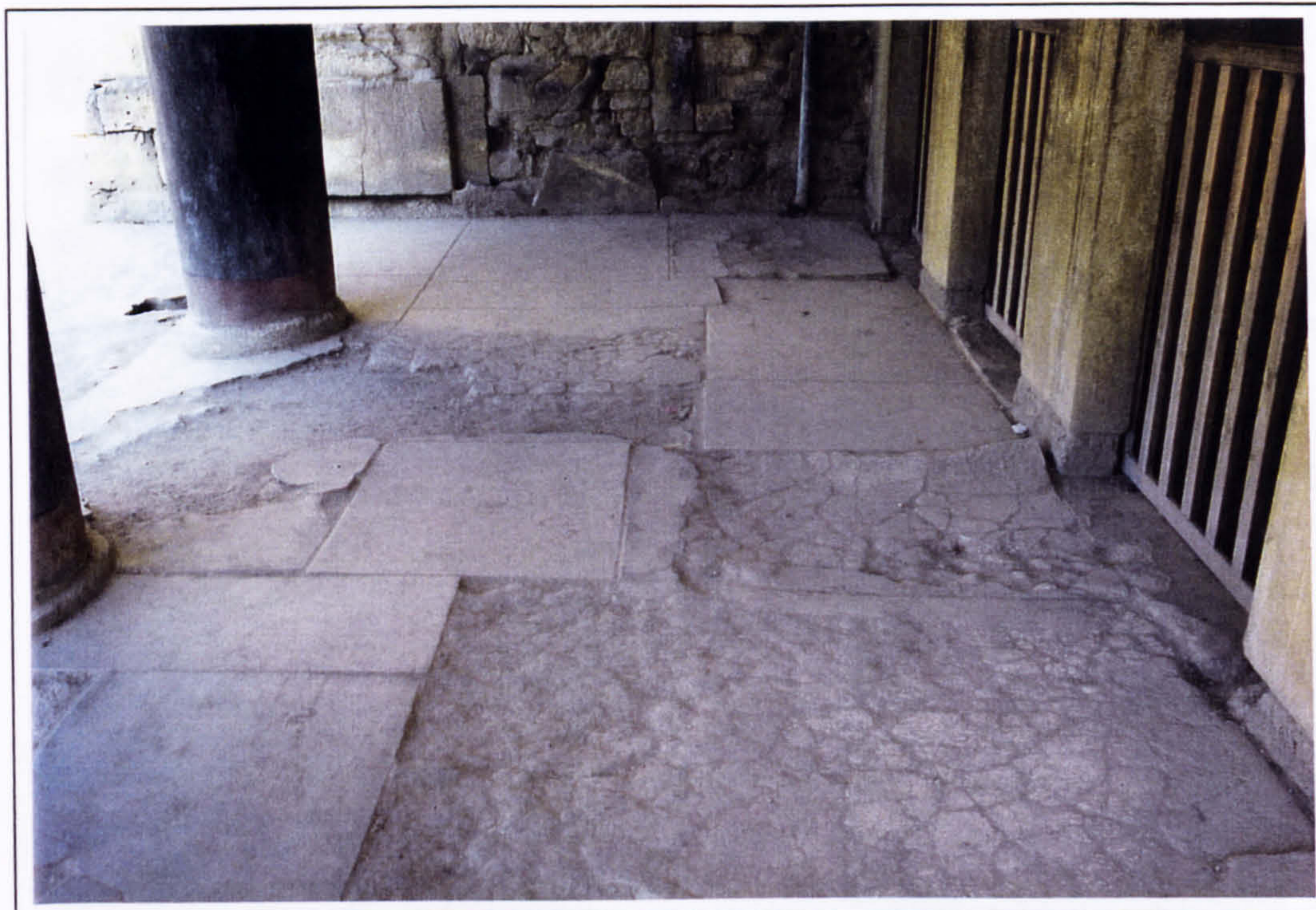
Plate 152 Decayed floor slabs and concrete repair slabs in the southern portico of the Hall of the Double Axes in 1997.
