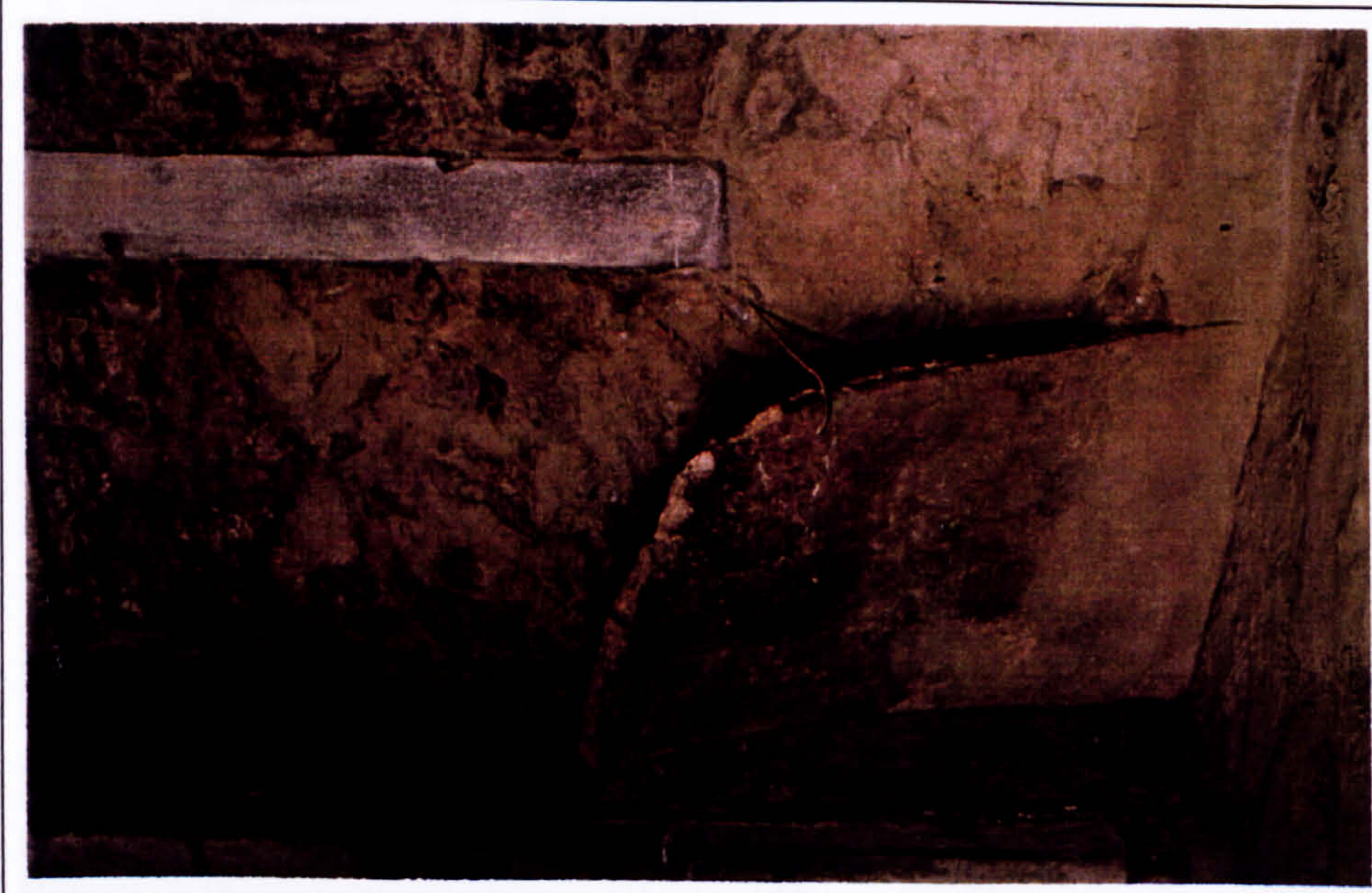
Plate 172 Warped gypsum dado in the Room with the Plaster Couch.
