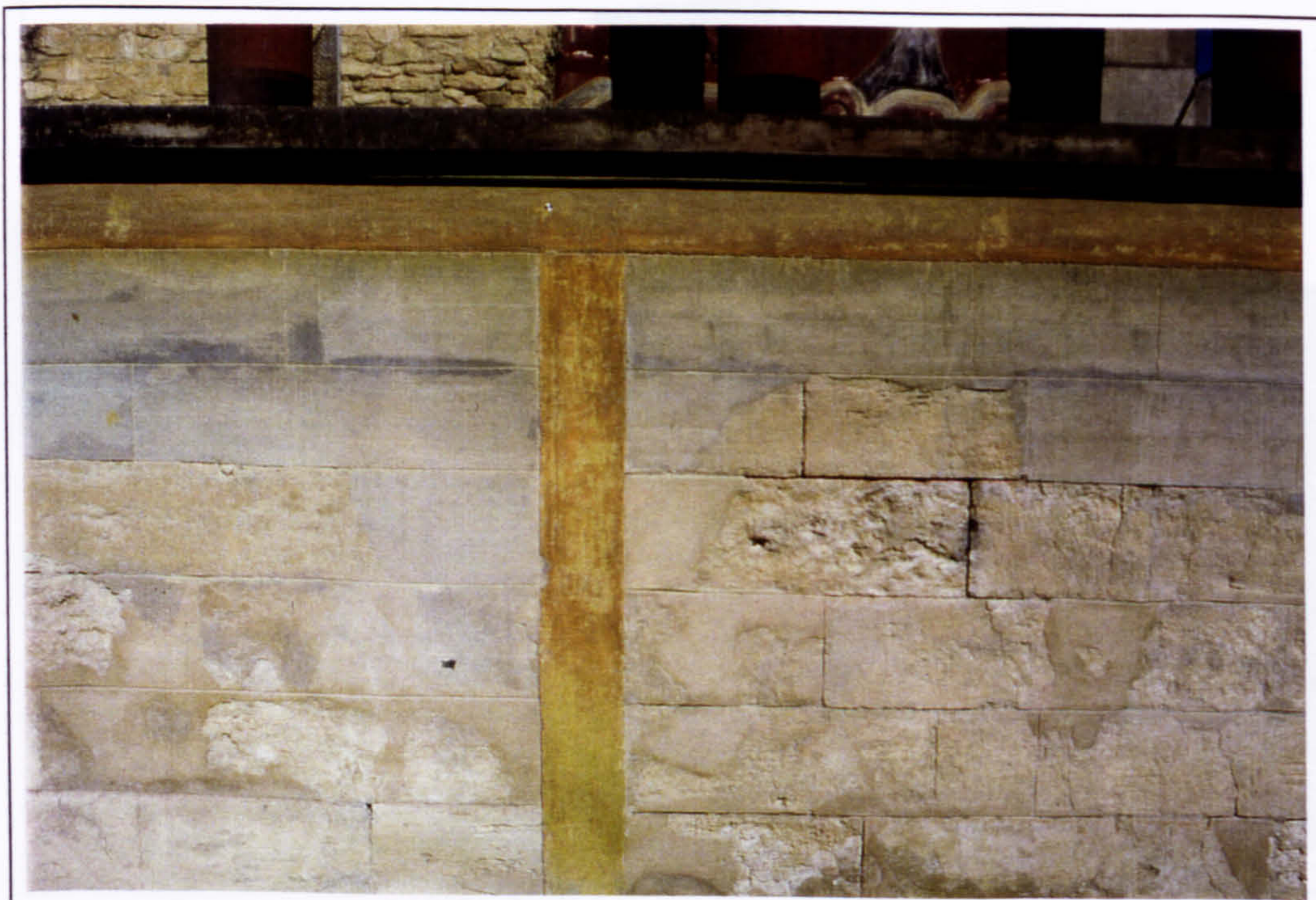
Plate 84 Detail of the original and reconstructed masonry of the North Entrance Passage's bastion in 1997.
