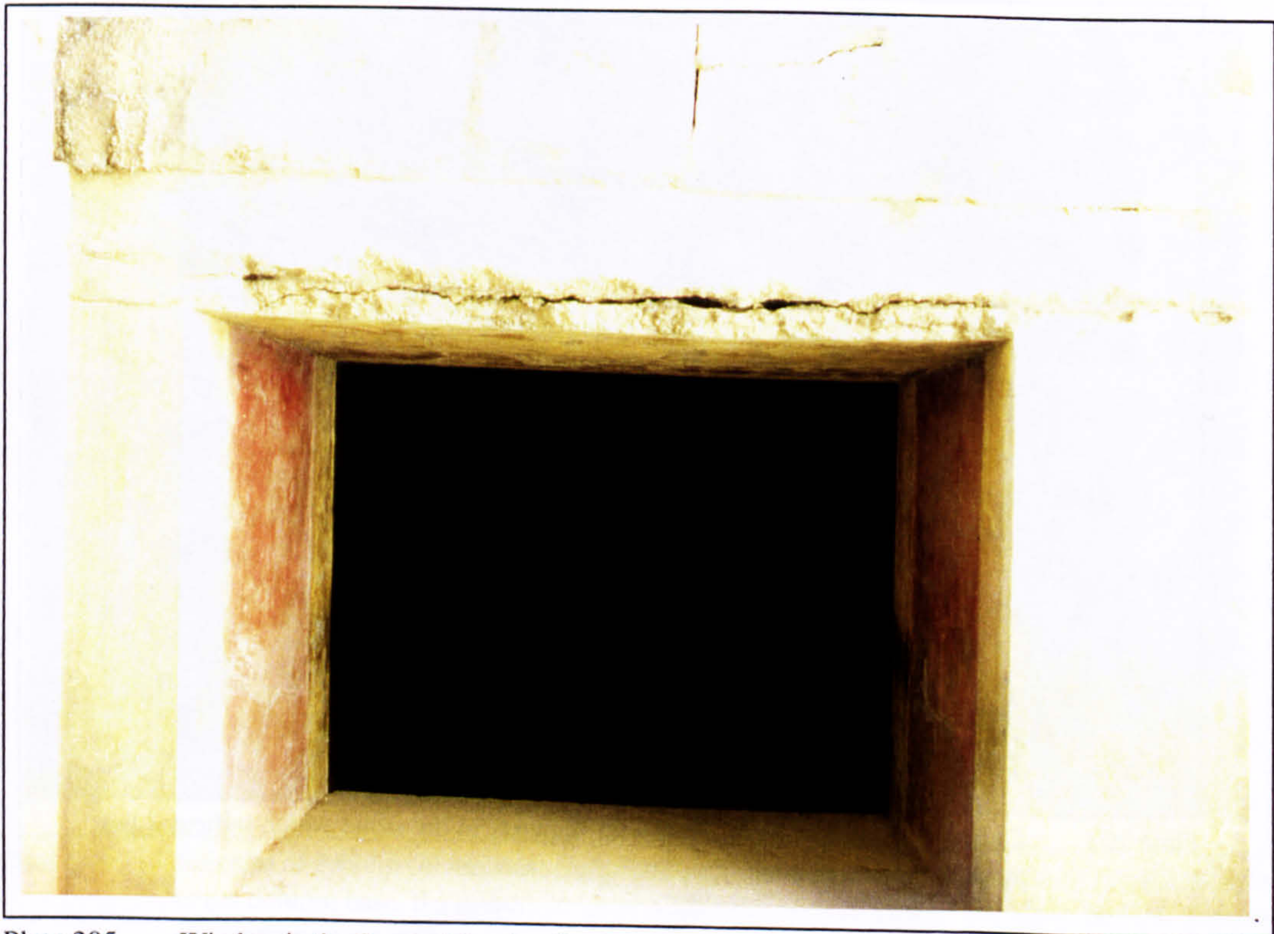
Plate 205 Window in the Court of the distaffs with rusting iron-I-beams exploding the concrete envelope.
