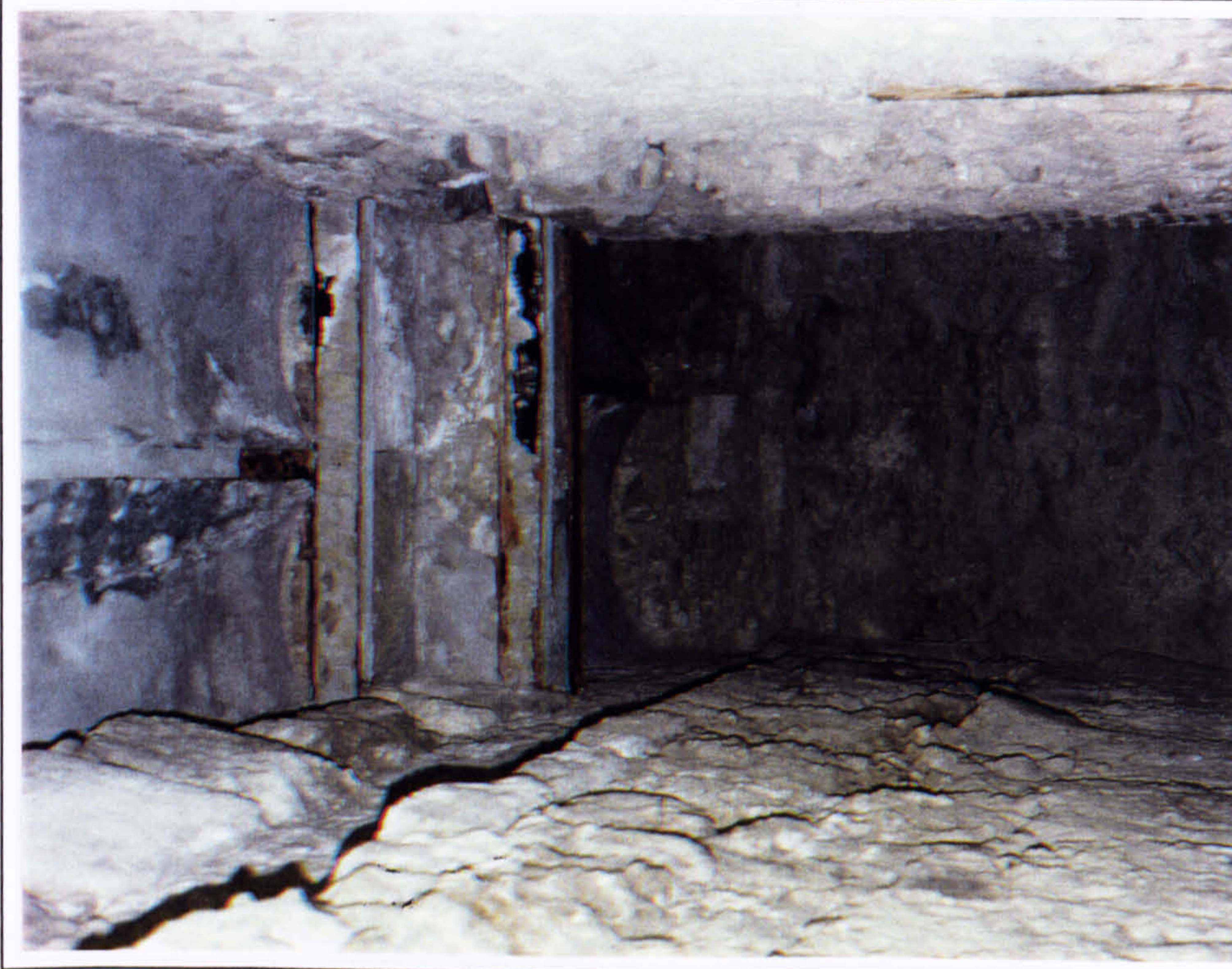
Plate 209 Ceiling of the Corridor of the Painted Pithoi wit water damage because of open joints in the paving above.
