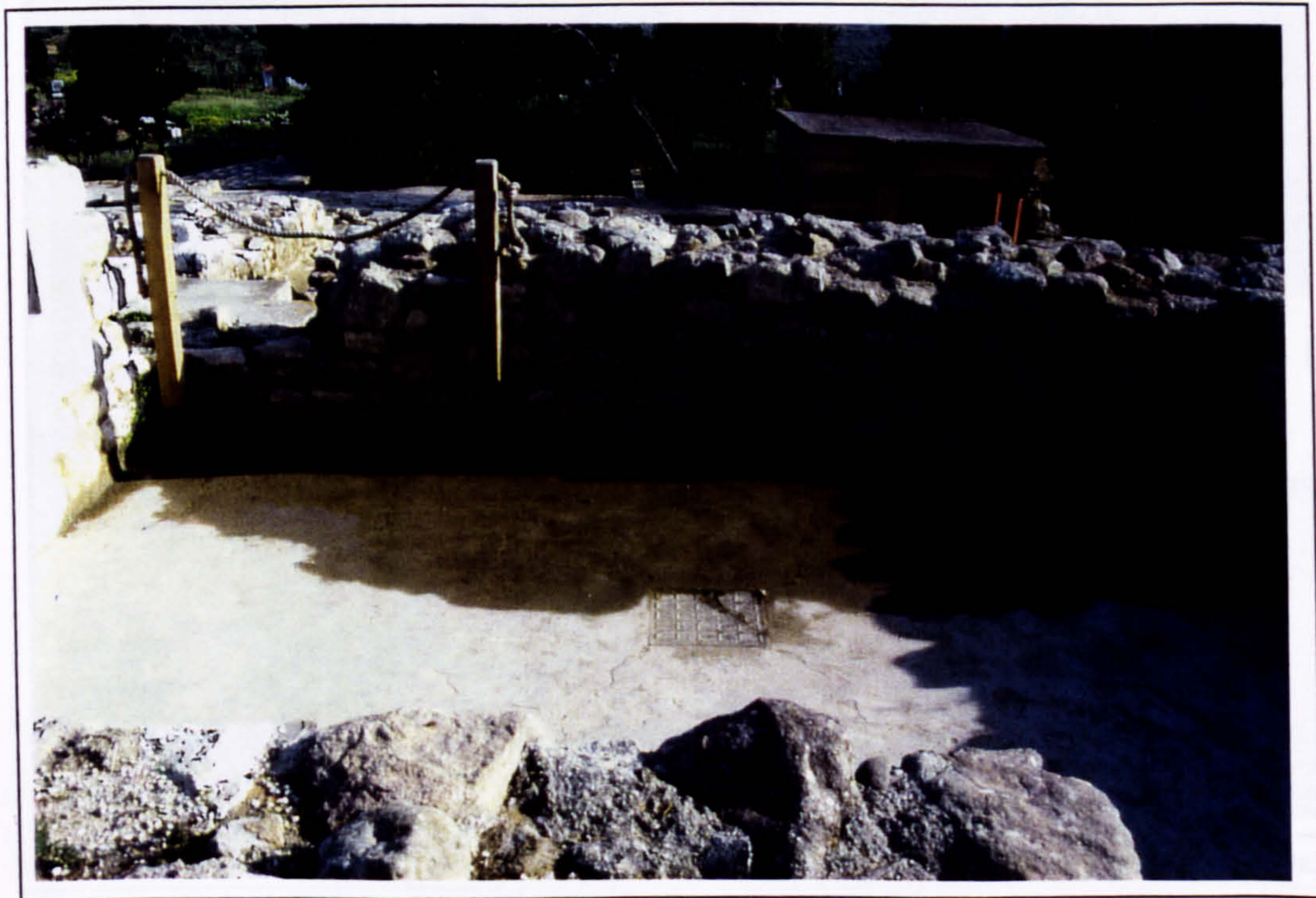
Plate 68 Water puddle at first floor of the reconstructed Throne Room indicating incline to drain rain-water. Puddle is due to blocked gaps in the walls.
