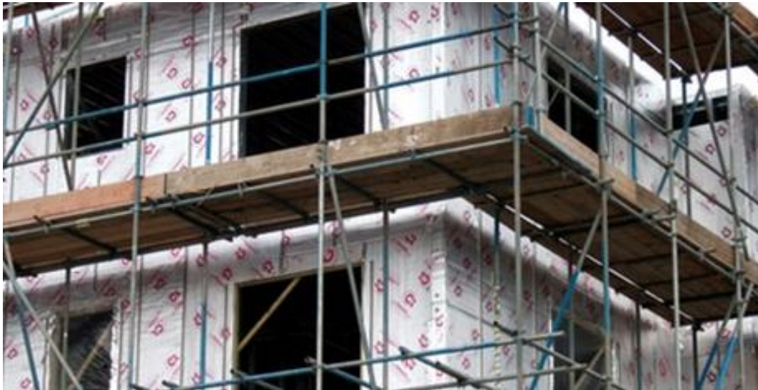
Figure 1.3: A building coated in metallic insulation such as Celotex could have a negative impact on expected propagation routes for wireless signals.
