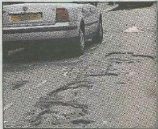
Struggle: potholes cost £68 each
