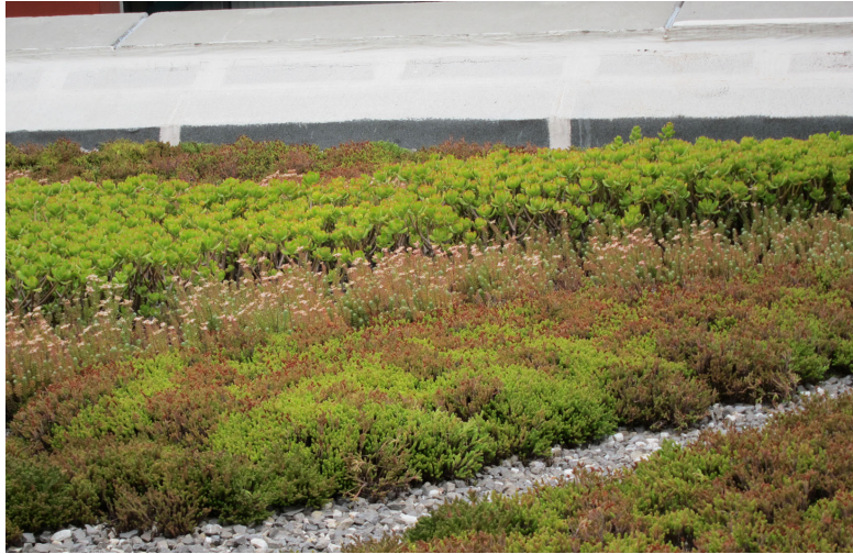
Figure 1.6.2 Green roof in roof of high school Felipe Carrillo Puerto in Mexico City with Sedum dendroideum , S. griseum and S. moranense .
