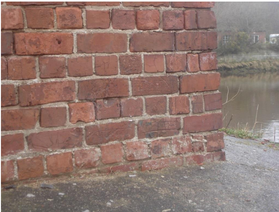
Figure F.6: Cracks on the outer faces of bricks, indicating spalling of face 1 surface.
