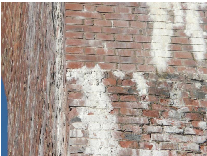
Figure F.2: Salt-damp defect on the top 9m of the pier, present on both repair and unrepaired parts.
