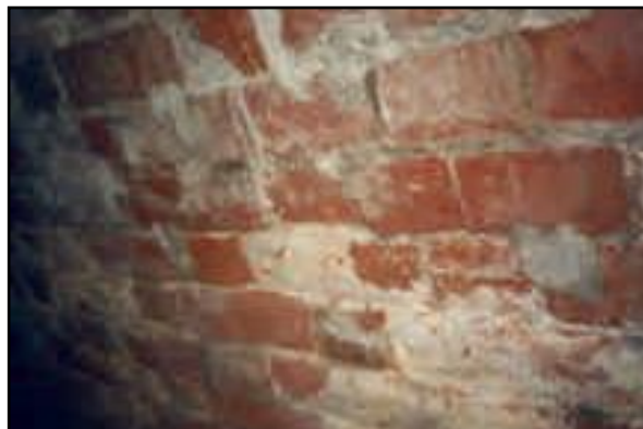
Figure 2.12: An example of efflorescence and crypto-florescence (Harrison, 1998).
