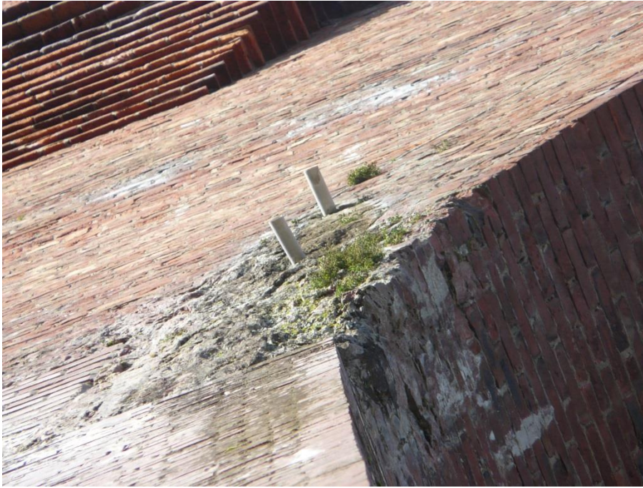
Figure F.5: The eroded zone around the drainage section on face 4 of the pier, showing plant growth close to the drainage pipes.
