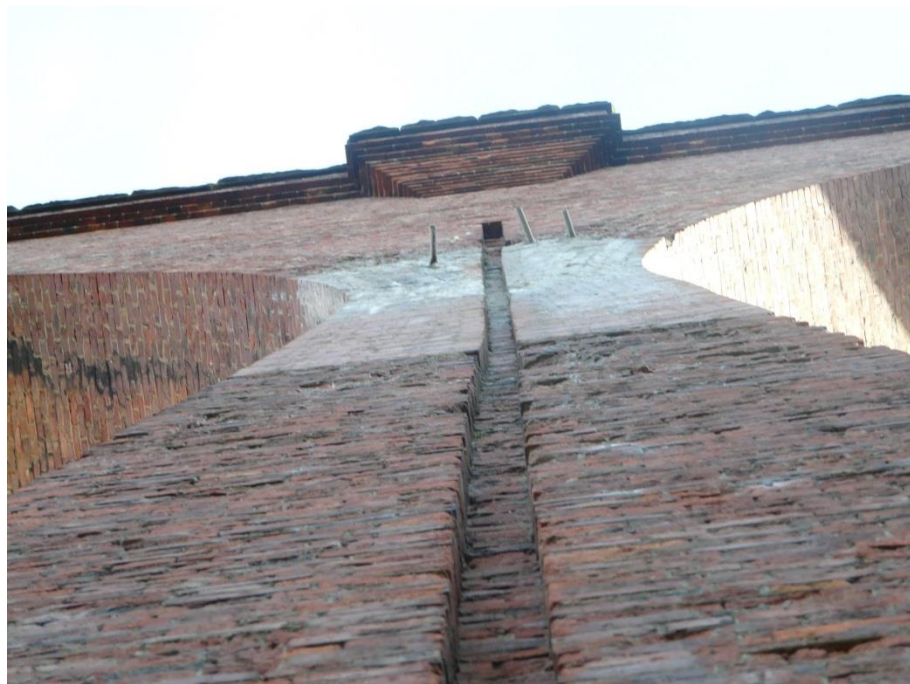
Figure F.4: Face 4 of the pier, different between the repaired and unrepaired section of the face.
