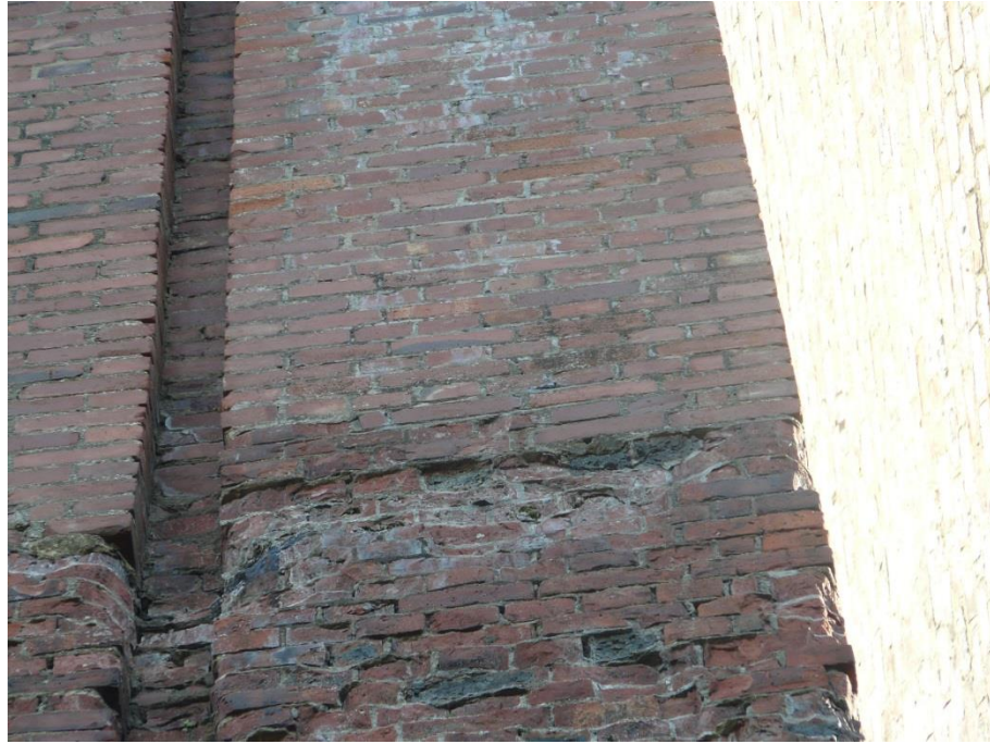
Figure F.3: Weathering defects causing exfoliation of stone on face 4 of the pier.
