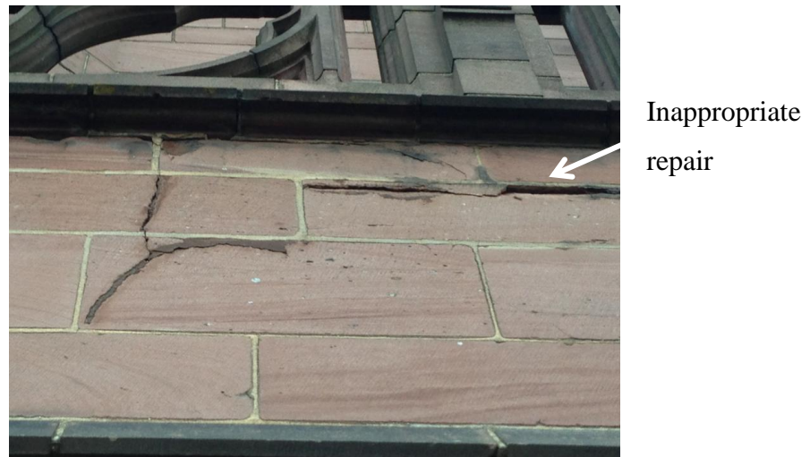
Figure 2.20: Inappropriate repair on the outer surface of the Liverpool Anglican Cathedral has caused further crack and damage.
