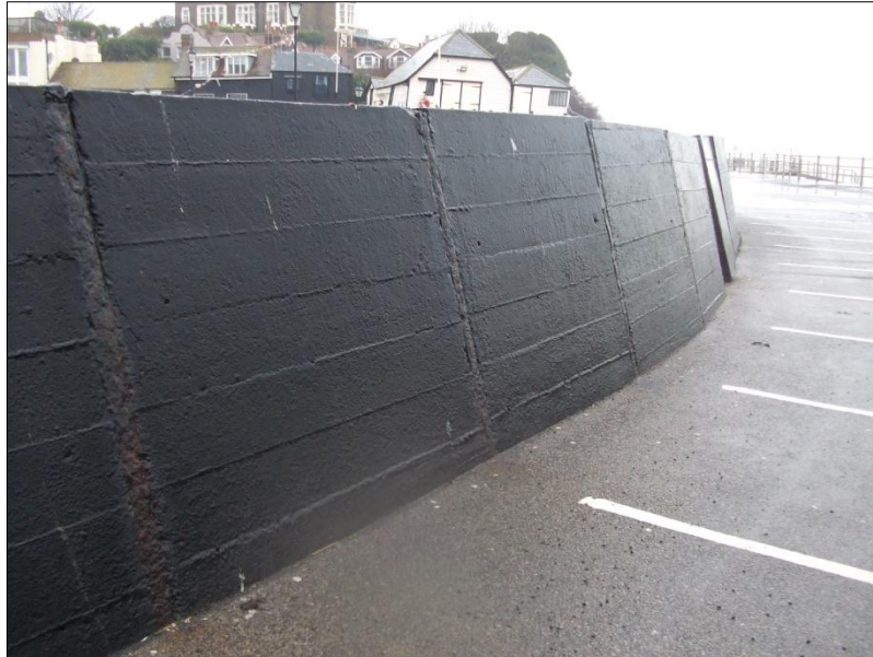
Figure 16, Detail of elevated walling (in position of former outer face of pier) now in concrete. Looking north
