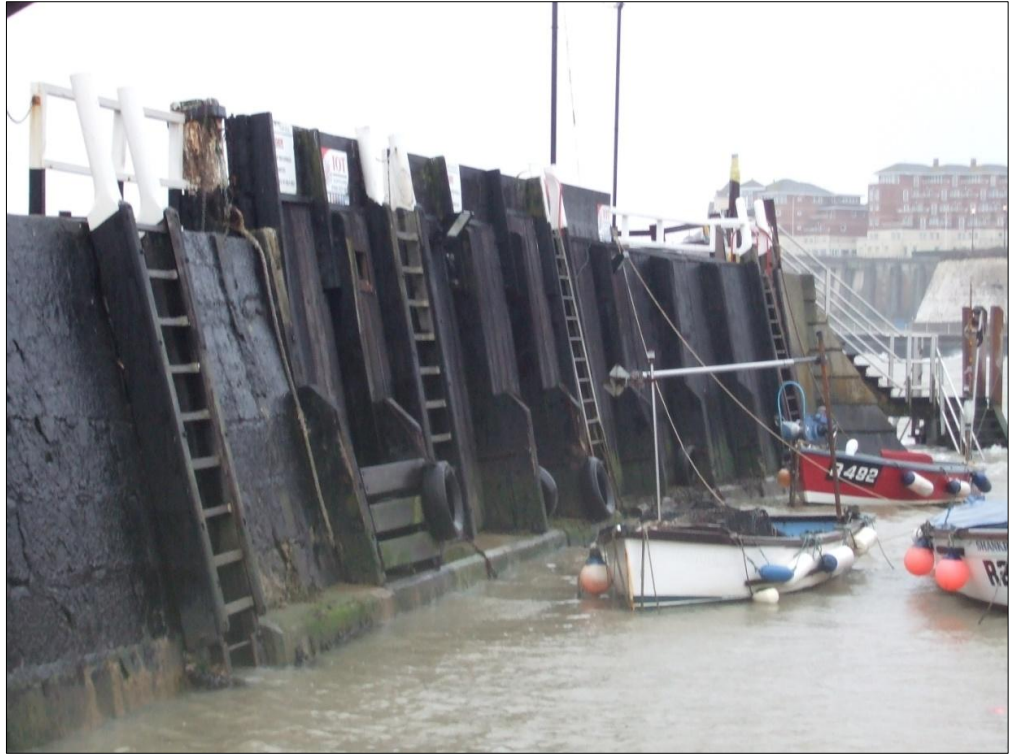
Figure 14, Timber to inner wall adjacent to head of Broadstairs pier, looking south
