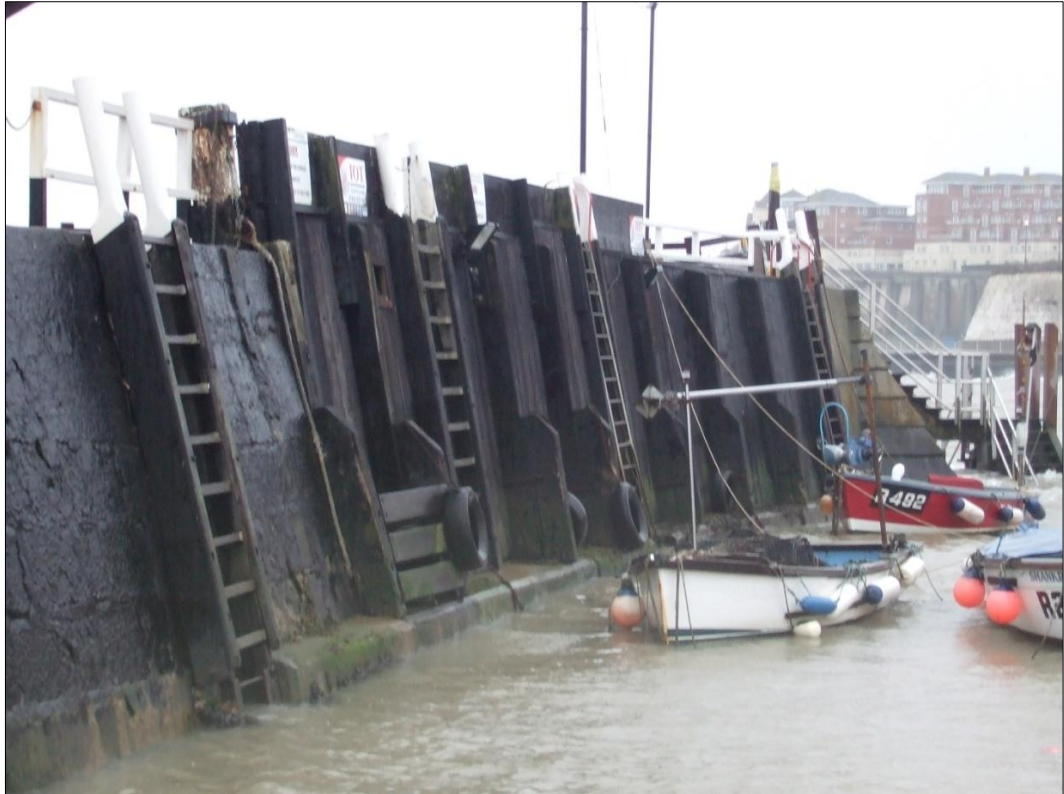
Figure 34, Broadstairs. Photograph of timber to inner wall of pier adjacent to head
