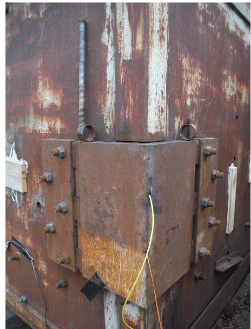
(d) Hinge secured, detonator shock tube (top) and breakwire seen protruding from hinge vertex
