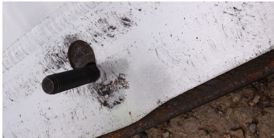
(c) Clamping bolt shank stretching panel hole
