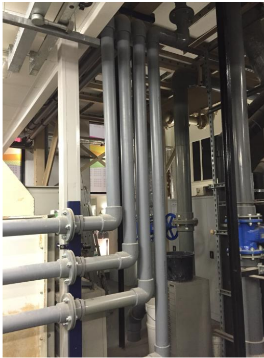
Figure 34– Connection between header tank and the three inlet pipes plus the inlet of the urban surface.
