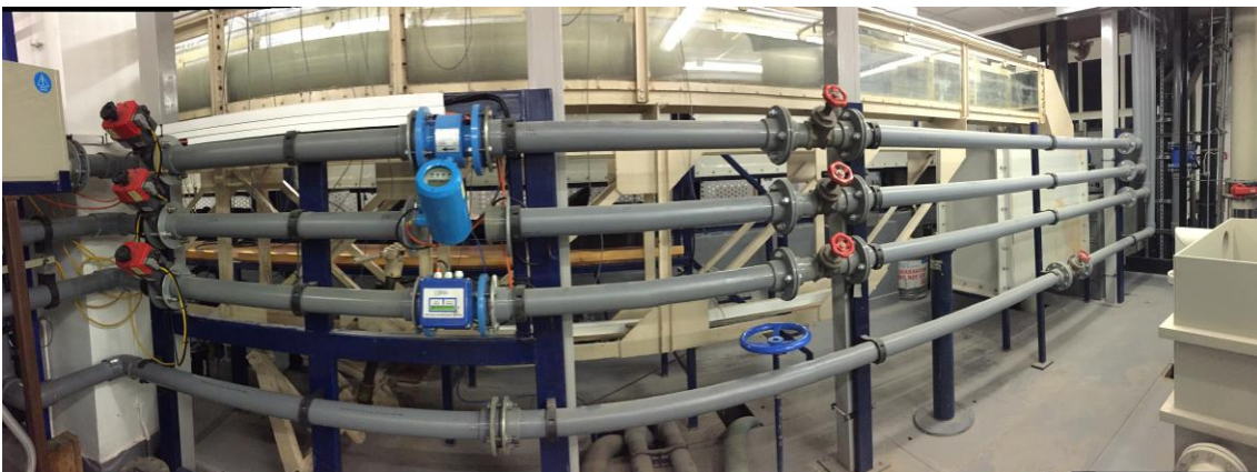
Figure 33 – Full view of the new inlet system.
