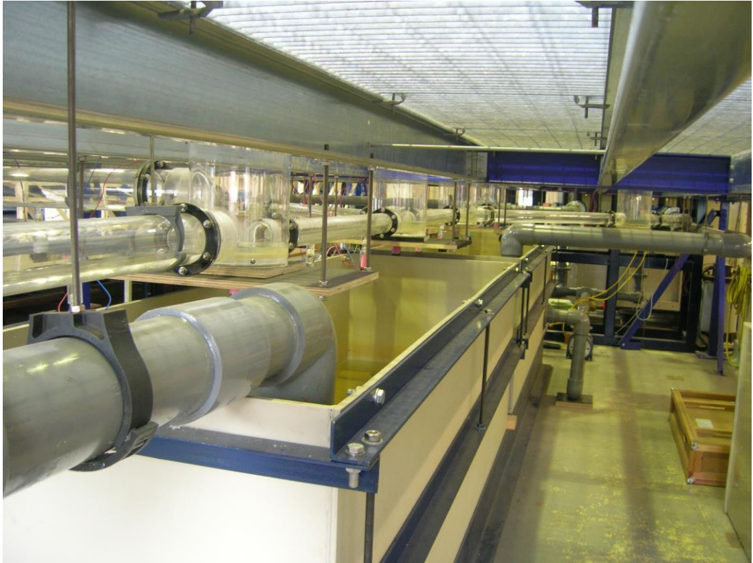
Figure 30 – Downstream view of the two re-circulating water tanks underneath the pipe system.
