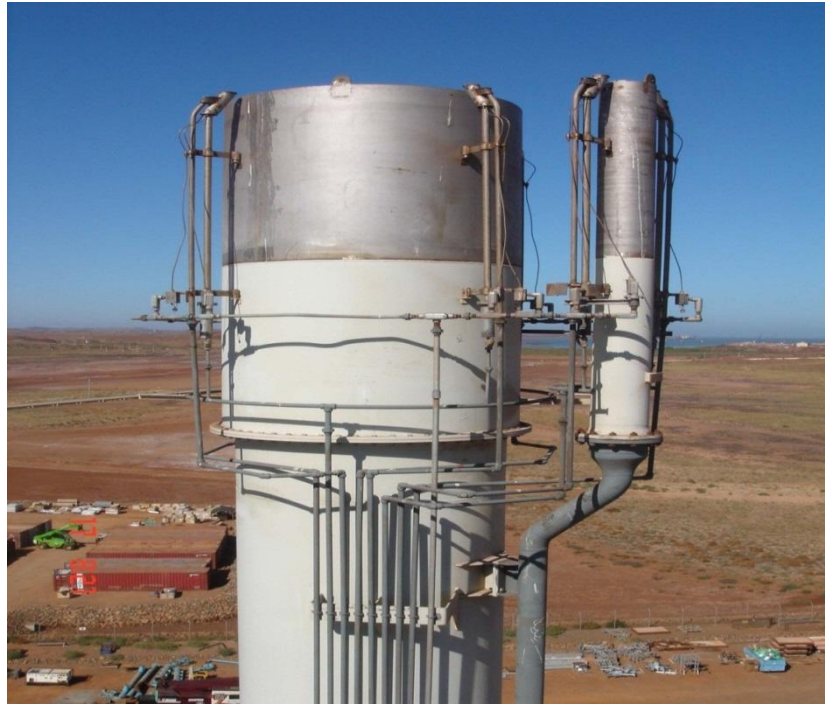
Figure 1-5 Photograph of a typical flare gas burner with pilot gas burners and a steam nozzle (adapted from Thermal Solutions Asia).
