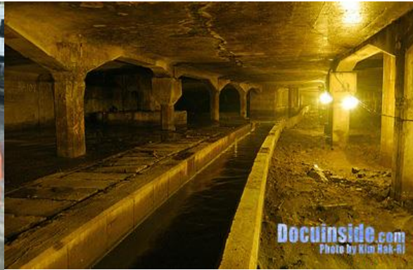
Figure 1.6 Under the covered CGC with full of a foul stench and rotten soil (Source: http://www.docuinside.com/ )
