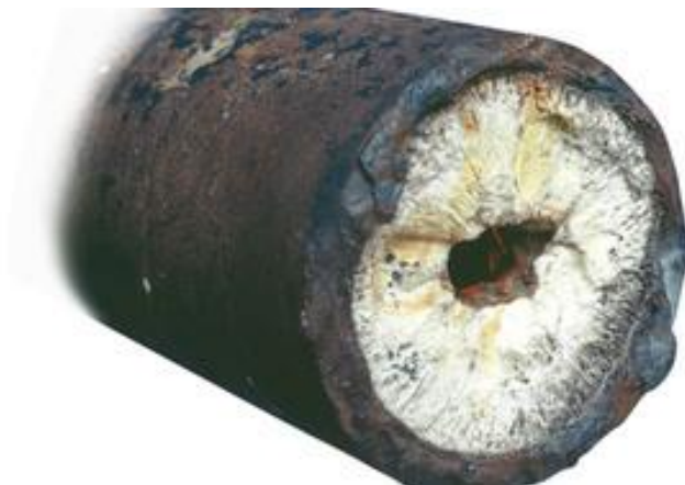
Figure 0-1. Image of mineral scale which has been formed inside the pipe (1)
