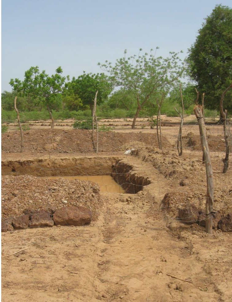
Figure 5.5 | On-farm runoff capture pond with conveyance canal (in progress – lining not in place), Ziga, Yatenga, Burkina Faso.
