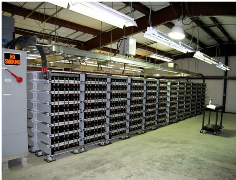
Figure 1.1 – A 1 MW/1.4 MWh BESS at Metlakatla Power & Light, Alaska. The installation consists of 378 Exide VRLA modules.
