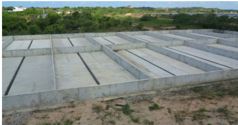
Figure 7.5 Construction of drying beds for microalgae cultivated in wastewater in Pium, RN, Brazil. Beds have a capacity for 4 tonnes algae to be dried per day, the algae currently retails for £25 per tonne
