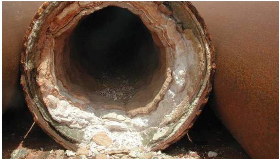
Figure 1.2: Limescale deposition in a pipe [64].
