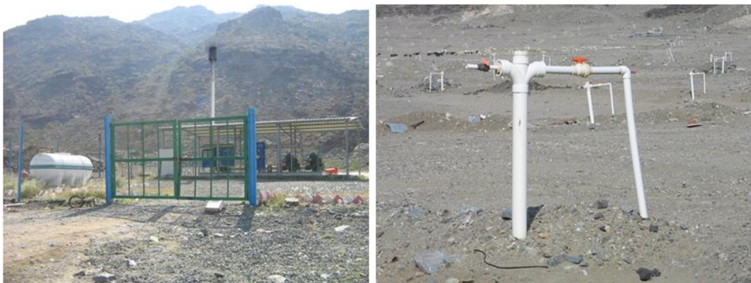
Figure 3. 25: Gas collection and burning flare of the old landfill in Makkah
