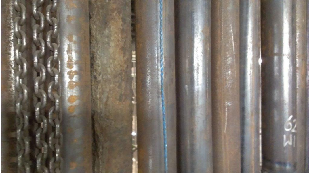
Figure 2.1 Photograph from a commercial boiler during plant shutdown showing corroded and replaced waterwall tubes.
