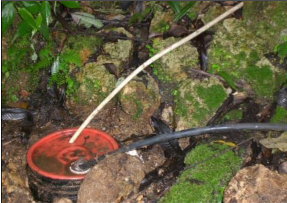
a) El Portillo water source consisting of a bucket and plastic pipes.
