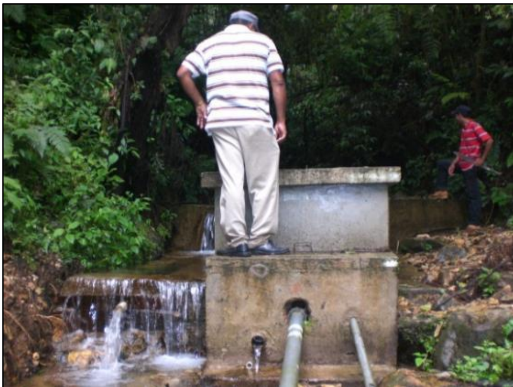
d) Closed box-style water source of La Labor community, with overflow at left-hand side.
