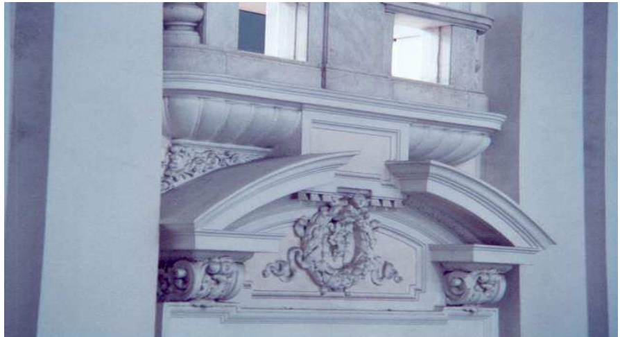
5.62. Interrupted gable decorated with flowers and mouldings. Source from Shue and Huang, 2003.
