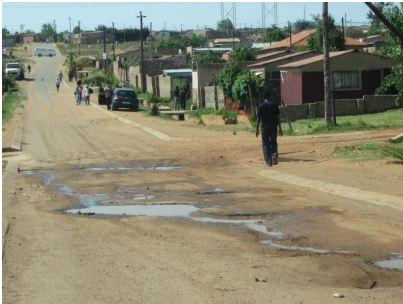
Figure 8-1: Poorly maintained roads in Bramfischerville (author’s own 2011).
