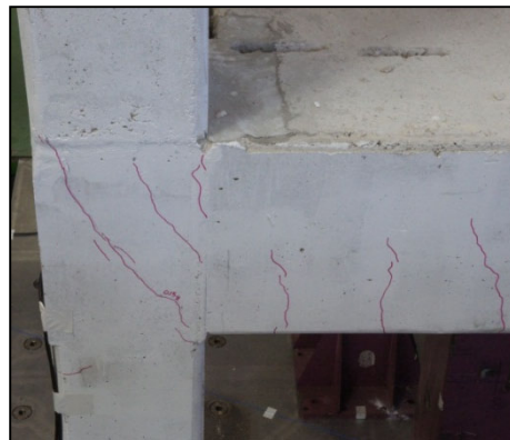
Figure 11-12: Damage of joint J1A-1 st at 0.15g – bare structure
