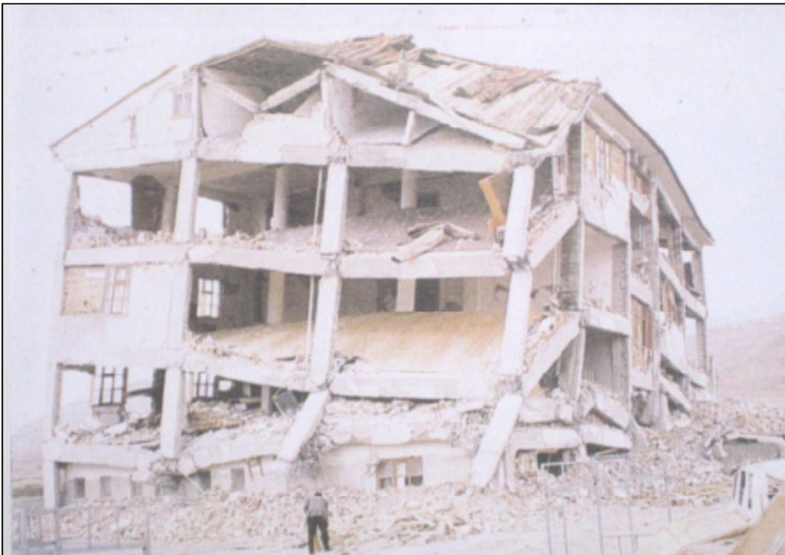
Figure 1-1: Connection failure and partial building collapse in the March 13, 1992, Erzincan, Turkey, earthquake (Hassan, 2011)
