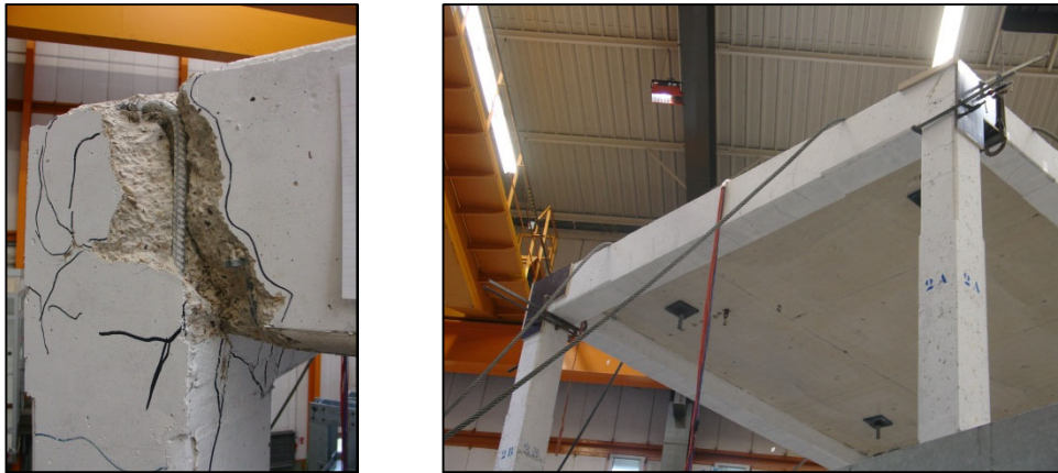
Figure 11-3(a): Concrete debris removal (left) and joint shoring after casting with new repair mortar (right)
