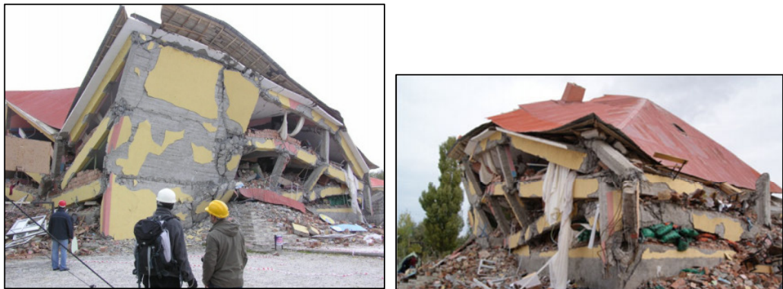
Figure 1-3: Total collapse of a three-story school in Turkey, partly due to rupture of joints (Erciş-Van, Turkey, earthquake of October 23, 2011)
