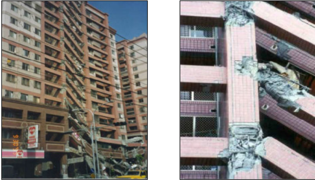
Figure 1-2: Partial building collapse and beam-column failure in Chi-Chi, Taiwan, earthquake of Sep. 21, 1999 (Uang et al., 1999)
