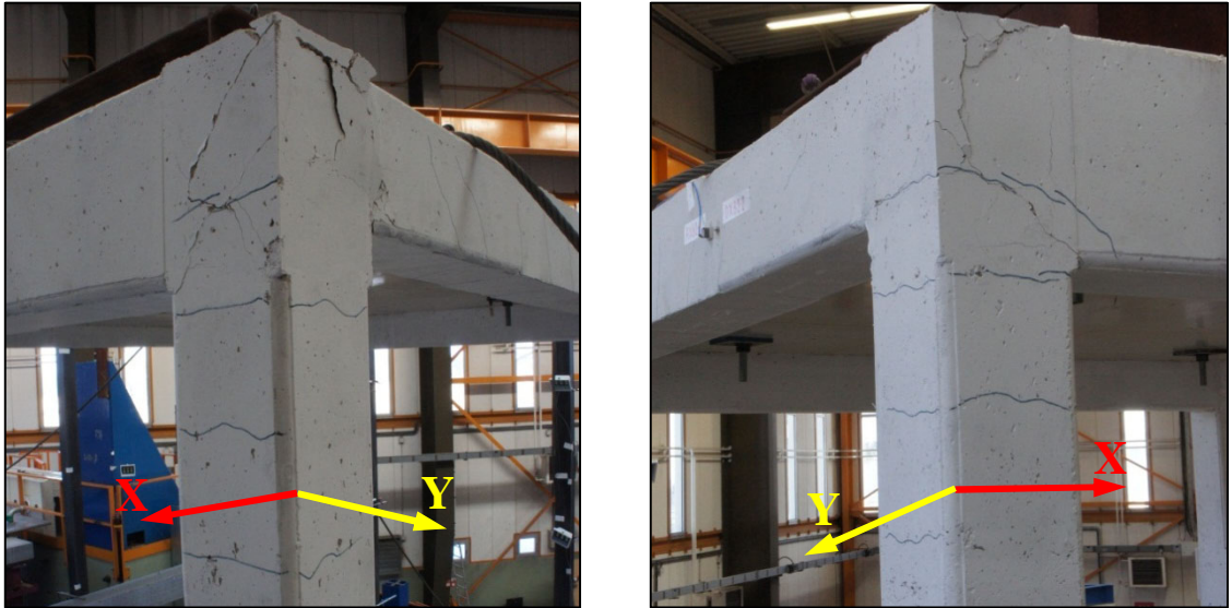
Figure 11-10: Damage of joint J2A-2 nd (left) and J2B-2 nd (right) at 0.15g – bare structure
