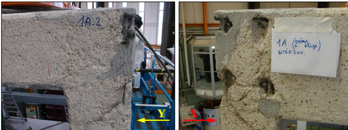
Figure 11-17: Damage of joint J1A-2 nd at 0.15g – second series
