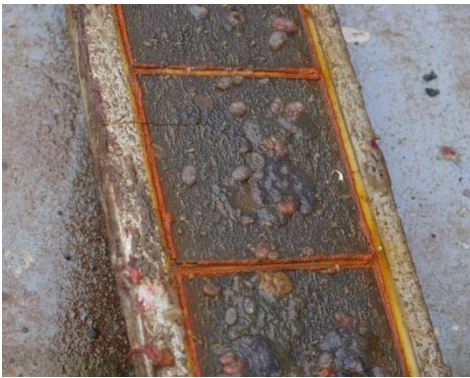
Figure 5.10. Corrosion and biofouling on panel D
