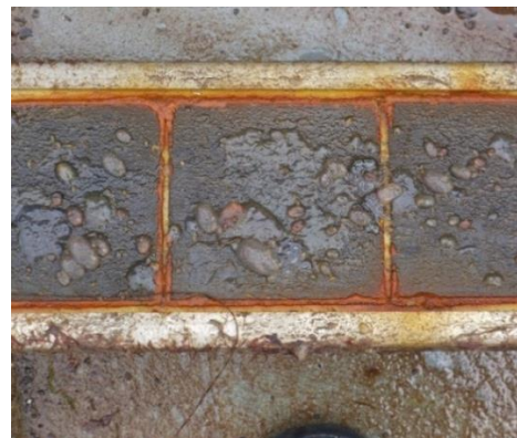
Figure 5.15. Corrosion and biofouling on panel I
