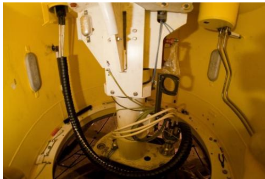
Figure 4.29. Anodic protection in the skirt area of the device
