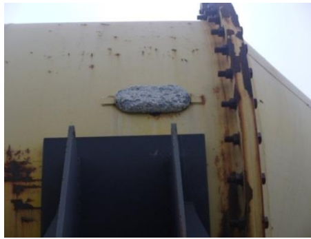
Figure 4.43. Corrosion on nacelle in small areas where protective paint has been removed
