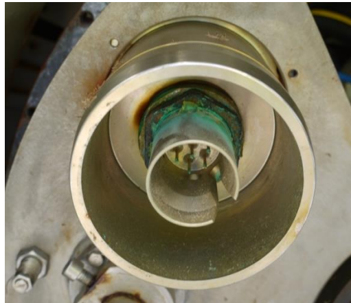
Figure 4.28. ADCP connector location on stab mechanism. Severe corrosion observed on the connector pins and around the base of the connector at the nut fixing
