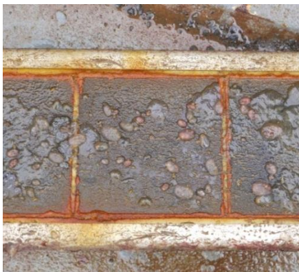
Figure 5.14. Corrosion and biofouling on panel H
