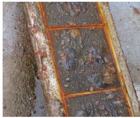
Figure 5.9. Corrosion and biofouling on panel C
