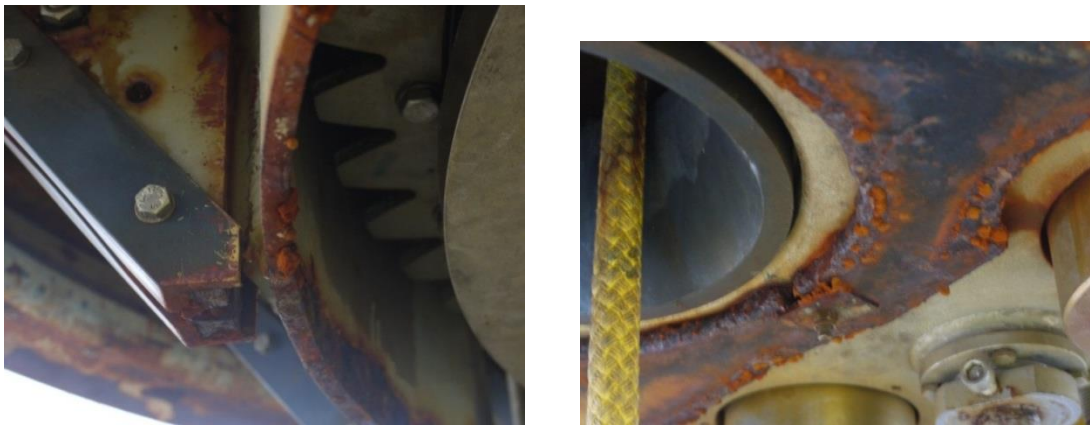
Figure 4.40 (a) and (b). Build-up of corrosion product in skirt
