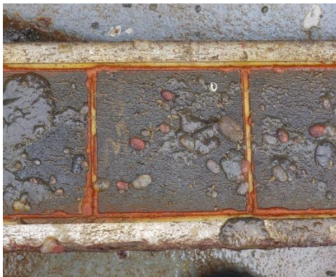
Figure 5.12. Corrosion and biofouling on panel F
