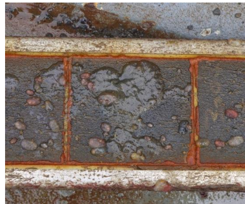
Figure 5.13. Corrosion and biofouling on panel G
