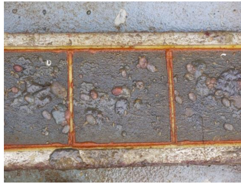
Figure 5.11. Corrosion and biofouling on panel E
