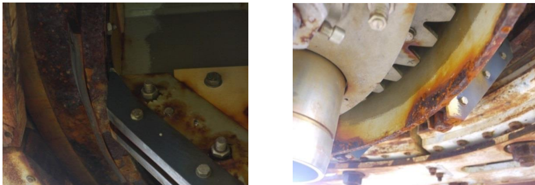
Figure 4.41 (a) and (b). Corrosion in skirt area and blistering of protective paint around fixings
