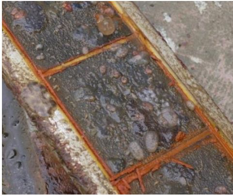
Figure 5.8. Corrosion and biofouling on panel B
