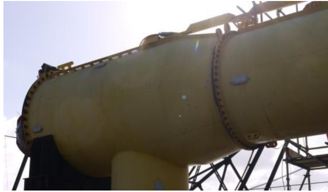
Figure 4.18. Paint flaking around flanges on Nacelle
