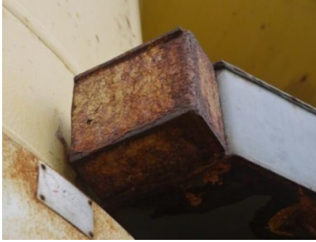
Figure 4.42. Corrosion on clamp equipment
