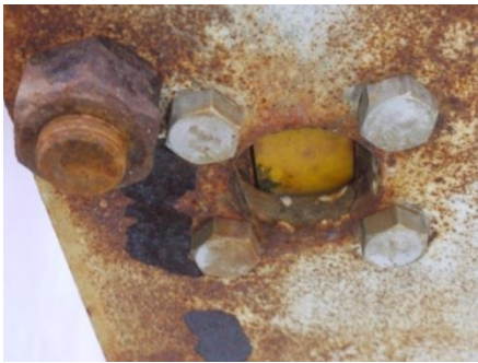
Figure 4.44. Corrosion and paint removal around fixings
