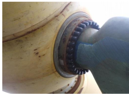
Figure 4.45. Corrosion around blade root fixings
