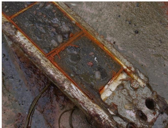
Figure 5.7. Corrosion and biofouling observed on panel A
