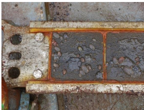
Figure 5.16. Corrosion and biofouling observed on panel J
