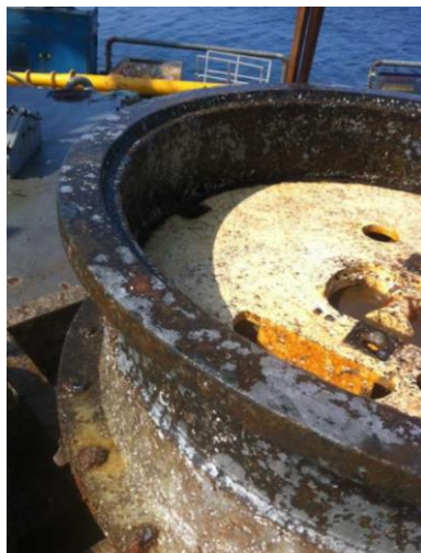
Figure 4.39. Flange after cleaning and removal of biofouling
