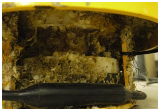
Figure 4.14. Fouling on the underside of the cartridge plate
