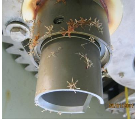
Figure 4.27. Corrosion and biofouling of the Seacon Hydralight fibre optic connector on the stab mechanism
