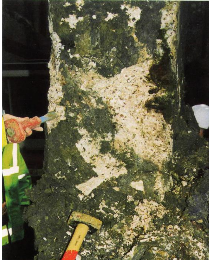
Figure 2.1 Example of thaumasite sulfate attack in highway bridge sub-structure BRE, (2005)
