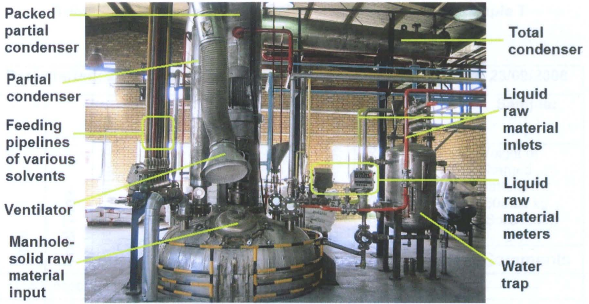
Figure 2.22 7000 litre reactor used for the industrial scale reproduction of sample T
