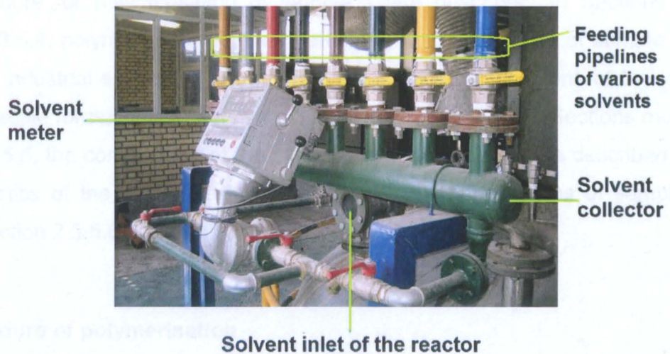
Figure 2.21 Solvent collector and solvent meter of the resin plant's twelve metric ton reactor
