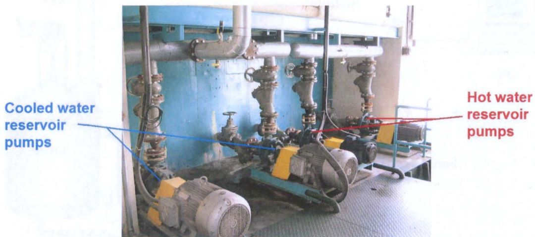
Figure 2.11 Pumps of the resin plant's water reservoir
