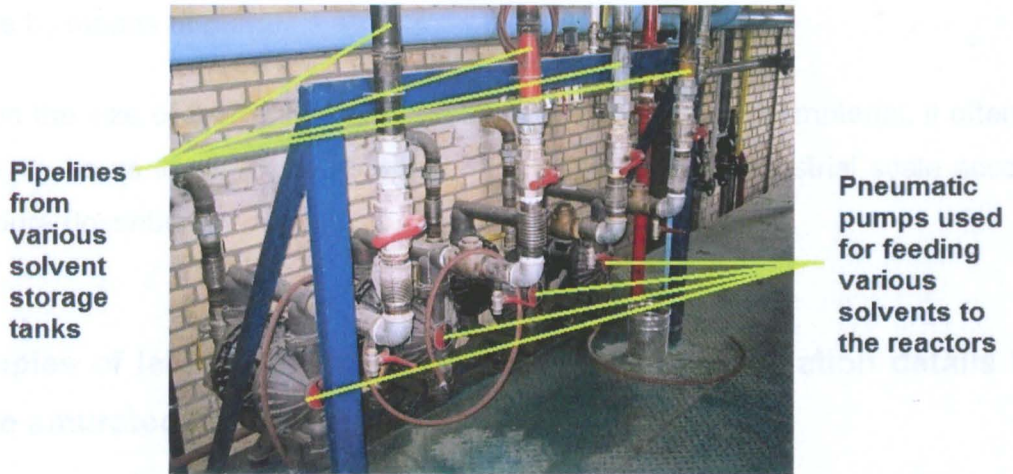
Figure 2.20 Pneumatic pumps of the solvent storage tanks of the resin plant
