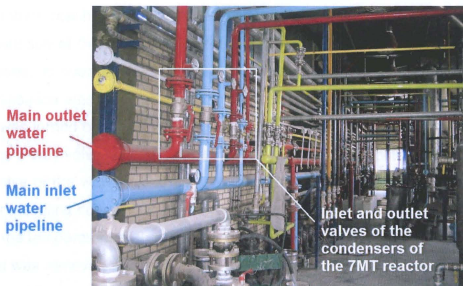
Figure 2.18 Main pipelines of the inlet and outlet water of the resin plant
