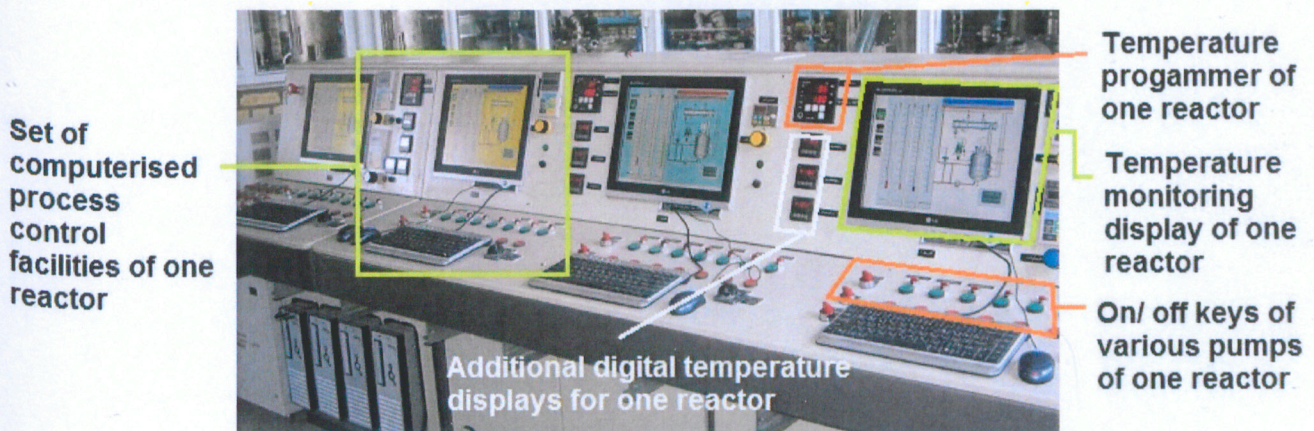
Figure 2.14 Temperature monitoring and process control room of the resin plant
