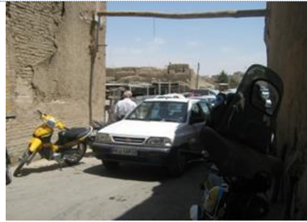
“The mud brick walls appear to be in a poor state of repair”
