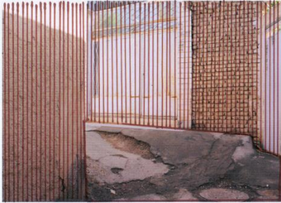
⚡ The pavement has really poor condition
