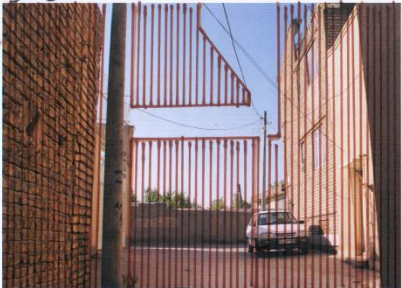
poor lighting design with a jumble of electricity cables
