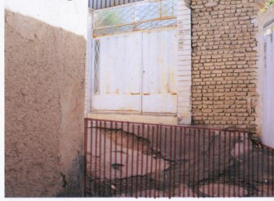
Really poor Buildings frontages on the both sides
