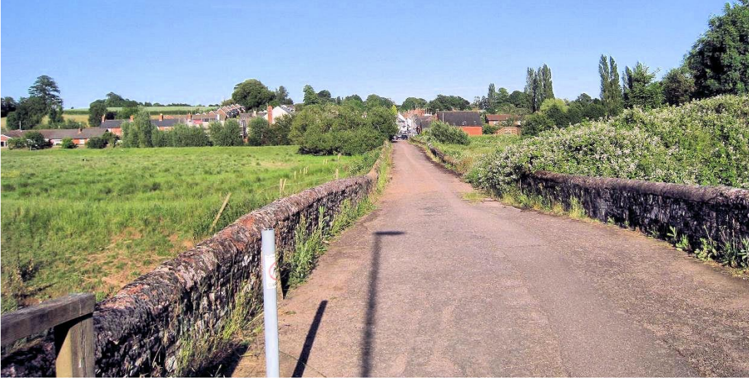
Fig.59. Photograph of Clyst Bridge looking east towards Bishop's Clyst. Note the length and narrowness of the bridge.
