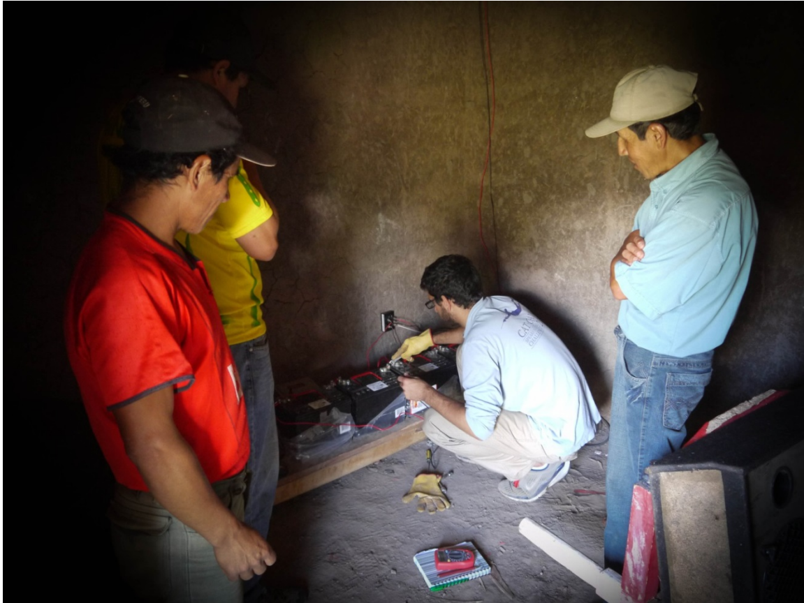
Figure 4-20: The two community members responsible for the wind turbine look on whilst WindAid staff rewire the inverter at El Olivo.
