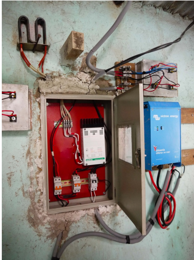
Figure 4-22: A much tidier and therefore easier to understand electrical system installed by Soluciones Prácticas.
