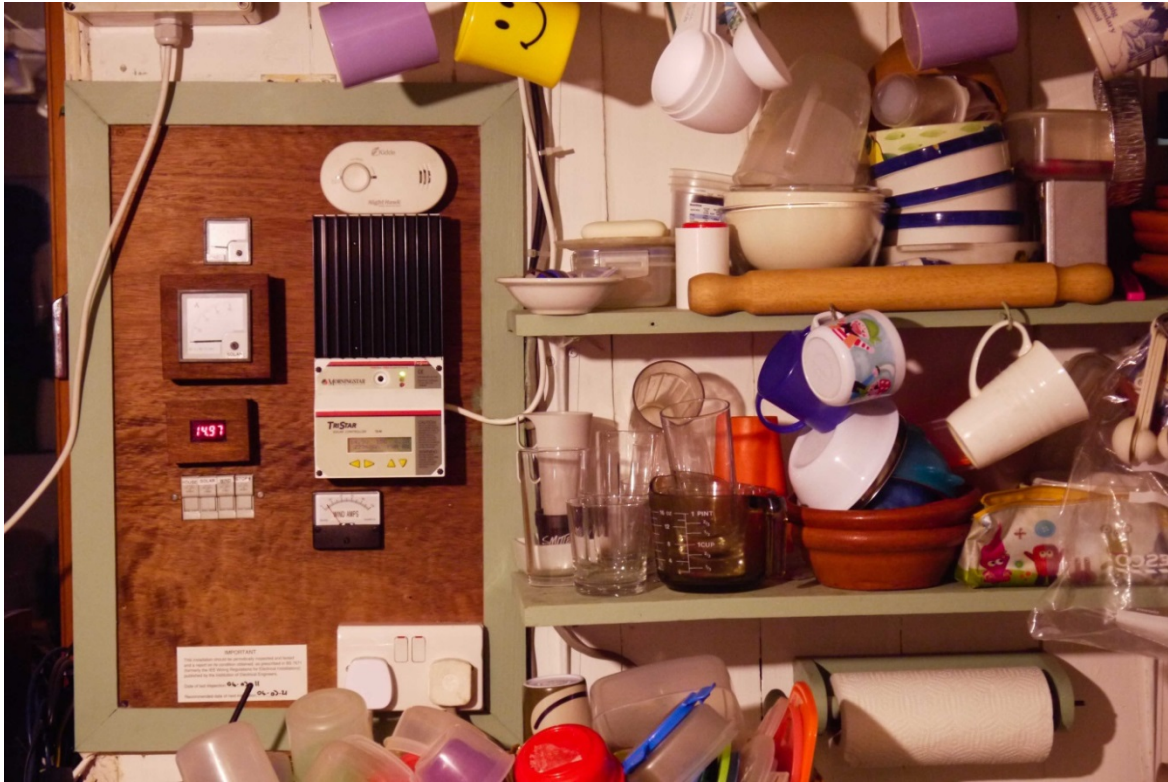
Figure 6-46: The battery voltage meter (and ammeters from the PV and wind turbines) neatly displayed in Andy and Susan's kitchen.
