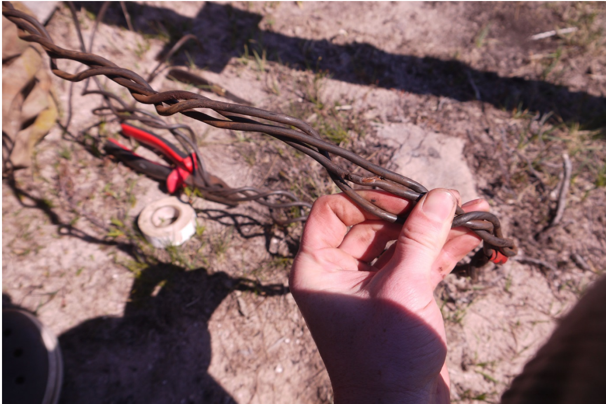
Figure A-10: The twisted power cable from inside the tower that was shorting out and stopping the turbine intermittently.
