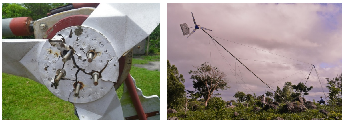
Figure 3-5: Transplanting a technology that was a) crumbling to pieces on the Caribbean coast of Nicaragua (blueEnergy, 2011) to b) the much more hospitable central highlands.
