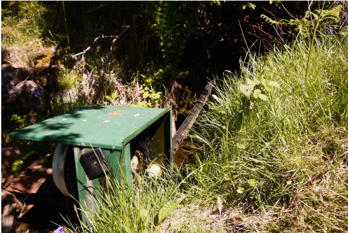
Figure 6-59: 200W EcolInnovation hydro turbine installed at the Brown residence.
