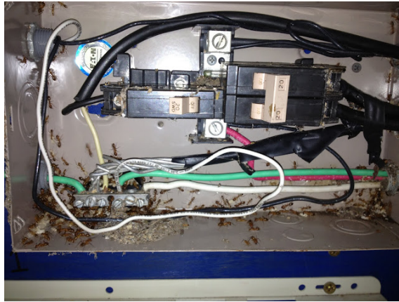
Figure 5-15: Invasion of the fuse box by ants that led to the failure of the solar controller in June 2012. Photo courtesy of Bryan Ferry.
