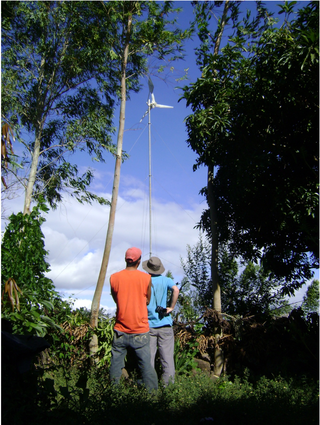
Figure 5-1: The author is shown the 1kW LMSWT that powers the remote community of Cuajinicuil in the central highlands of Nicaragua.
