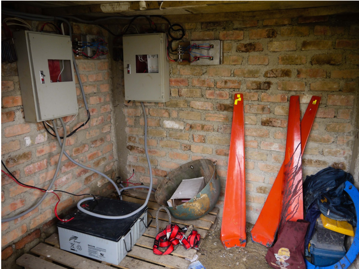
Figure 4-19: Toolbox, Spare blades, nose and other miscellaneous parts stored in the battery shed in Alto Perú (an even more extensive stock exists in El Alumbre).
