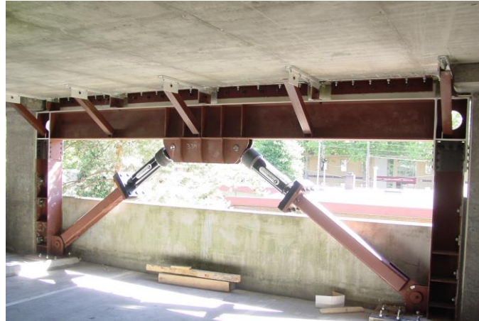
Figure 9: Damper been used in civil engineering to protect the structure from earthquake
