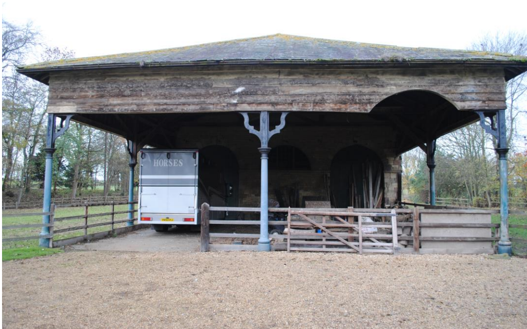
Figure 7. The loading bay at Thorp Arch. Note the columns and cut out compared to the picture below.
