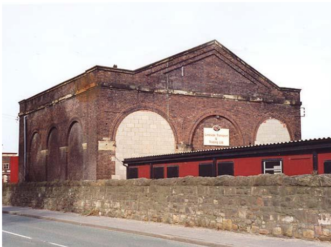
Figure 39. Mostyn goods shed in the 1990s, with stone course and rounded doors an obvious stylistic link to the sheds of Andrews. Courtesy of disused-stations.org.uk .
