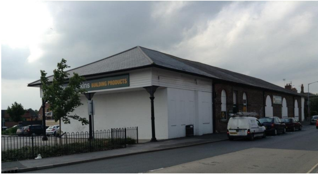
Figure 16. Pocklington goods shed showing the loading bay and extent of the original fabric of the shed.
