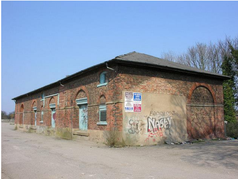
Figure 20. The outline of the demolished office is clearly visible at Cottingham. Courtesy of George Robinson.
