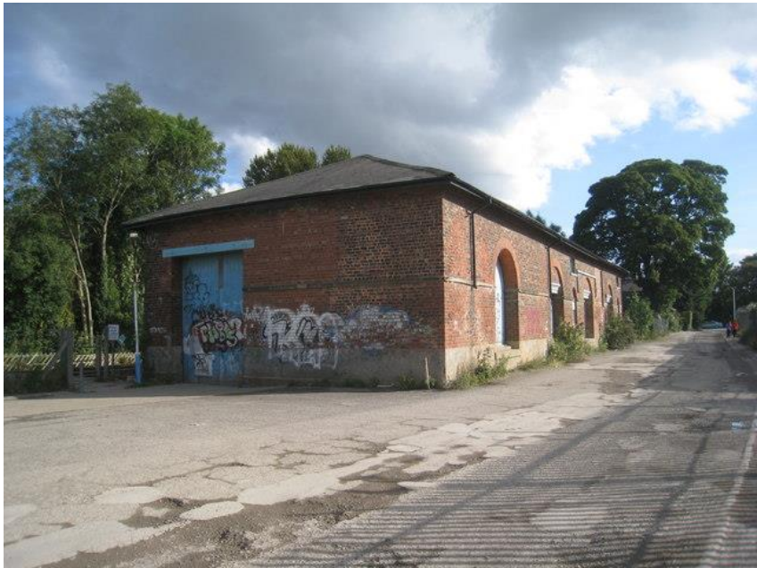
Figure 19. The road side of Cottingham goods shed, showing the surviving doors and windows. Courtesy of Jonathan Thacker.
