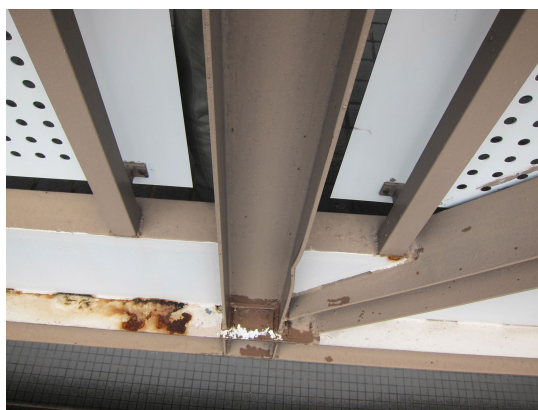
Figure 6-11. Rust and a dent in the flange of one of the vertical truss members at the centre of span B.
