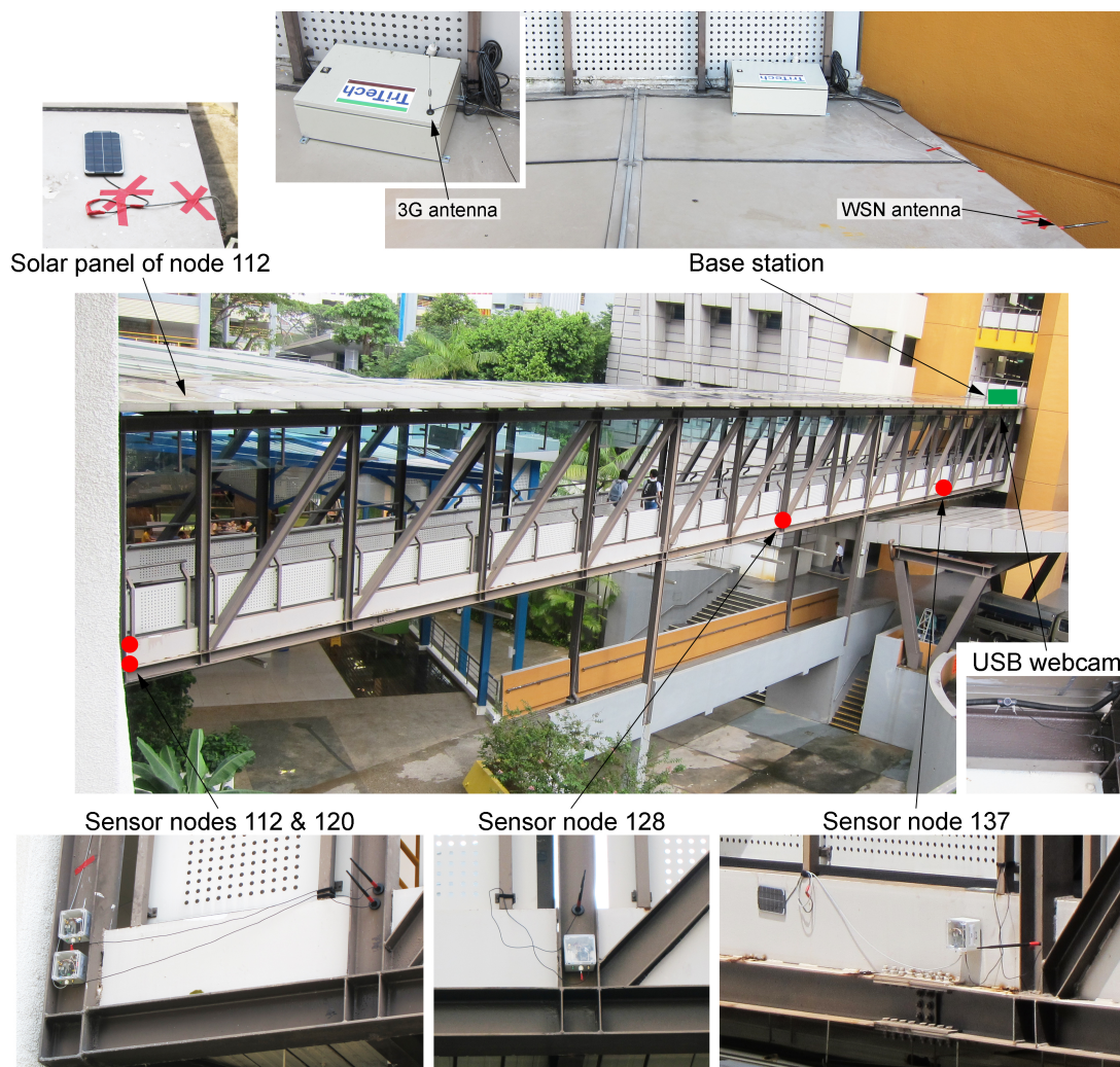
Figure 6-12. The wireless sensor network at the SPB.
