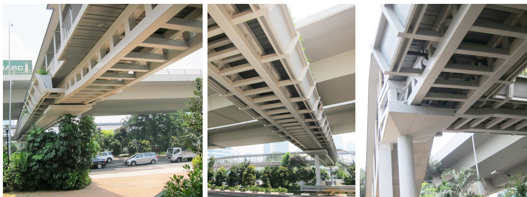
Figure 6-27. The POB truss structure of spans T6-T7 (left), spans T6-T5 (middle) and the connection between T4-T5 (right).
