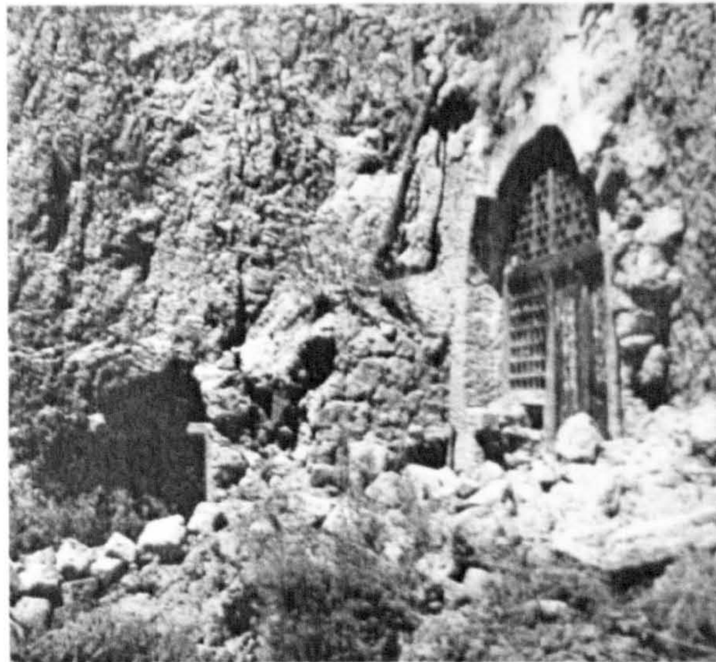
Figure 6.18 Collapsed cave dwelling after the flash flood of August 1963.
