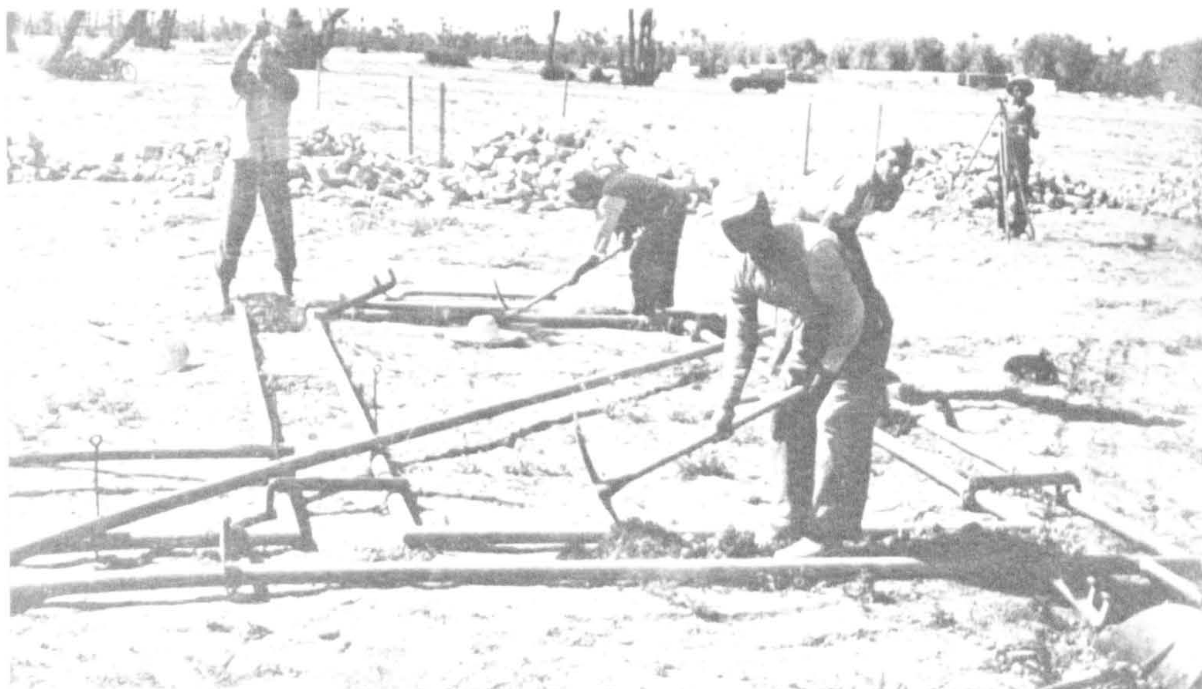
Template used for unskilled workers excavating earth for foundations of self-help houses. (1)
