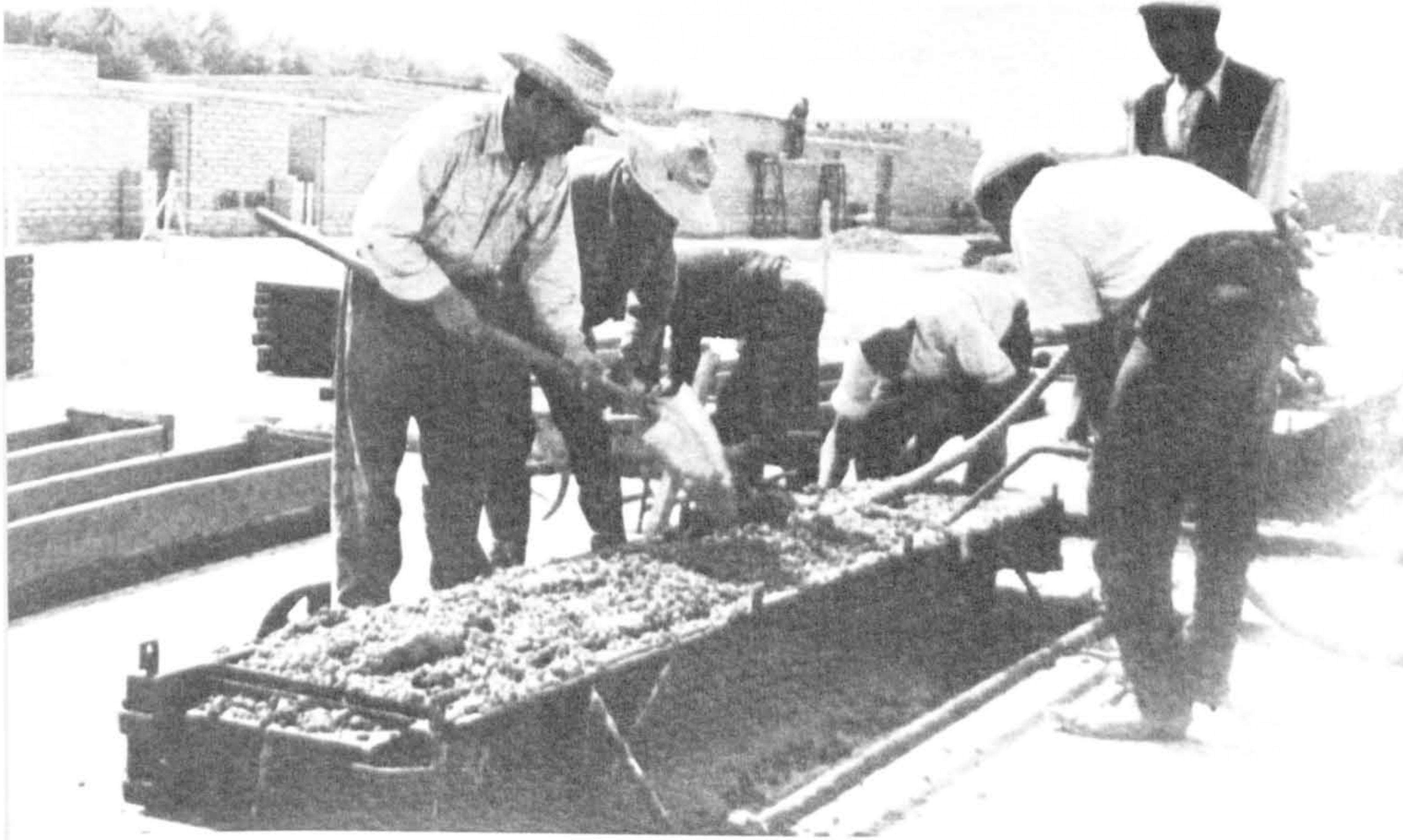
A sub-group preparing concrete beams while the rest of the group manages the brick laying.
