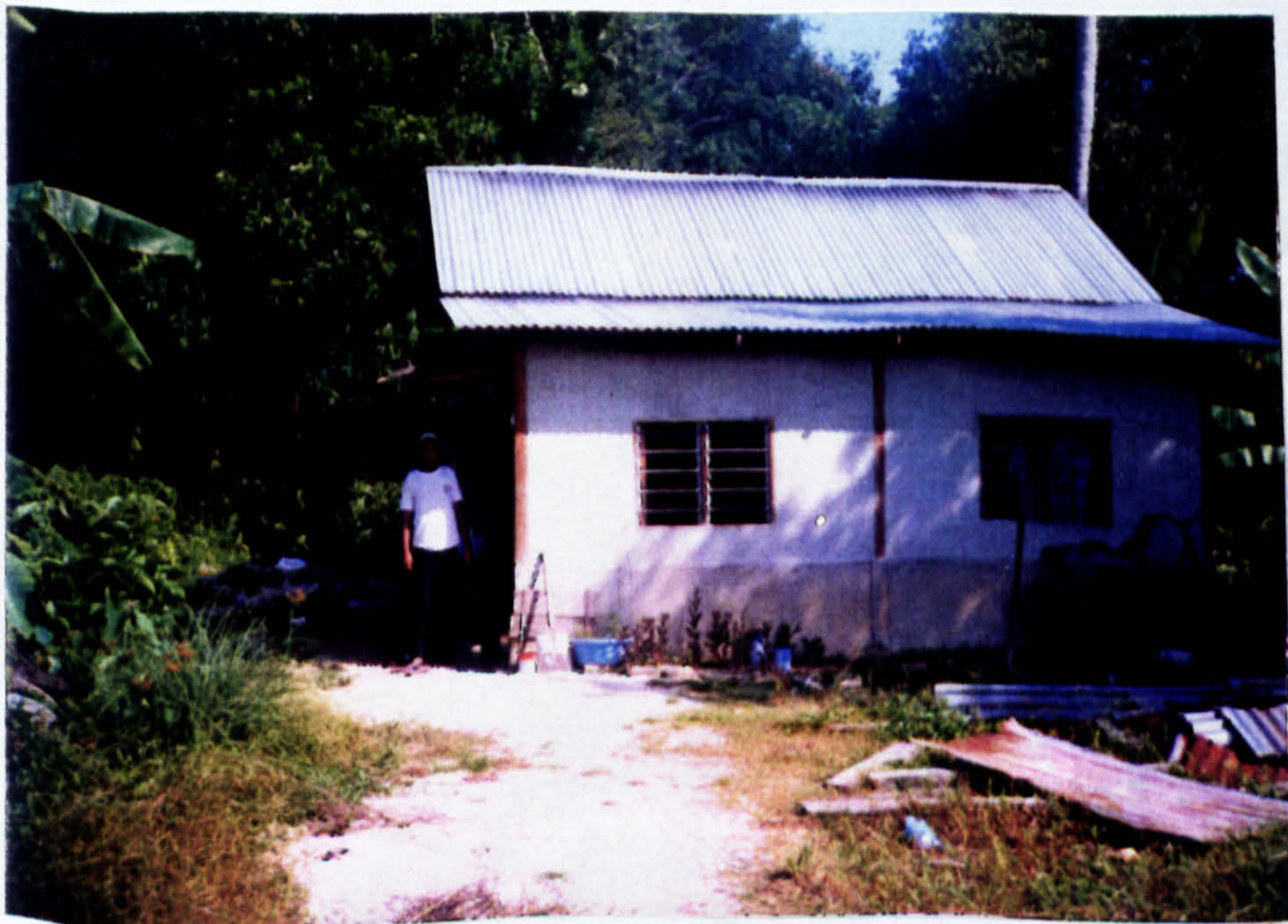
Plate O : House of peasant (single storey) : Cement wall and zinc roof. This type of house is generally seen as "firm" in terms of its structural condition.
