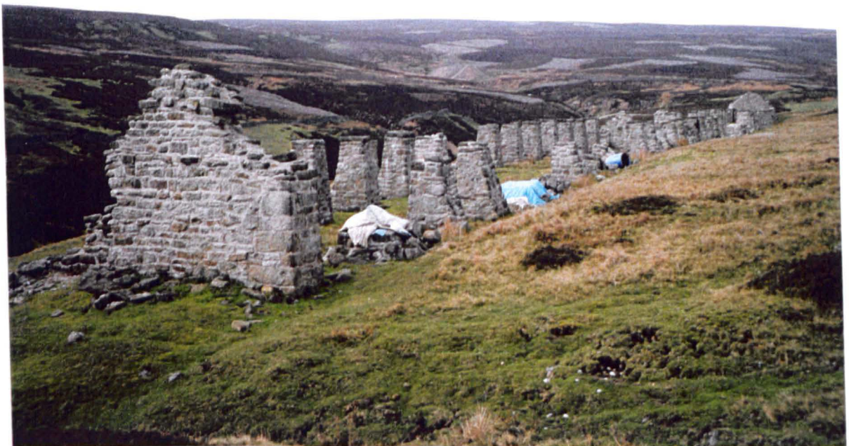
Fig. 4.8. The peat storage shed used by the Old Gang Smelting Mill, Swaledale. This structure, which is currently being renovated, is 119m in length and was open-sided and heather-thatched to facilitate the drying of the peat.
