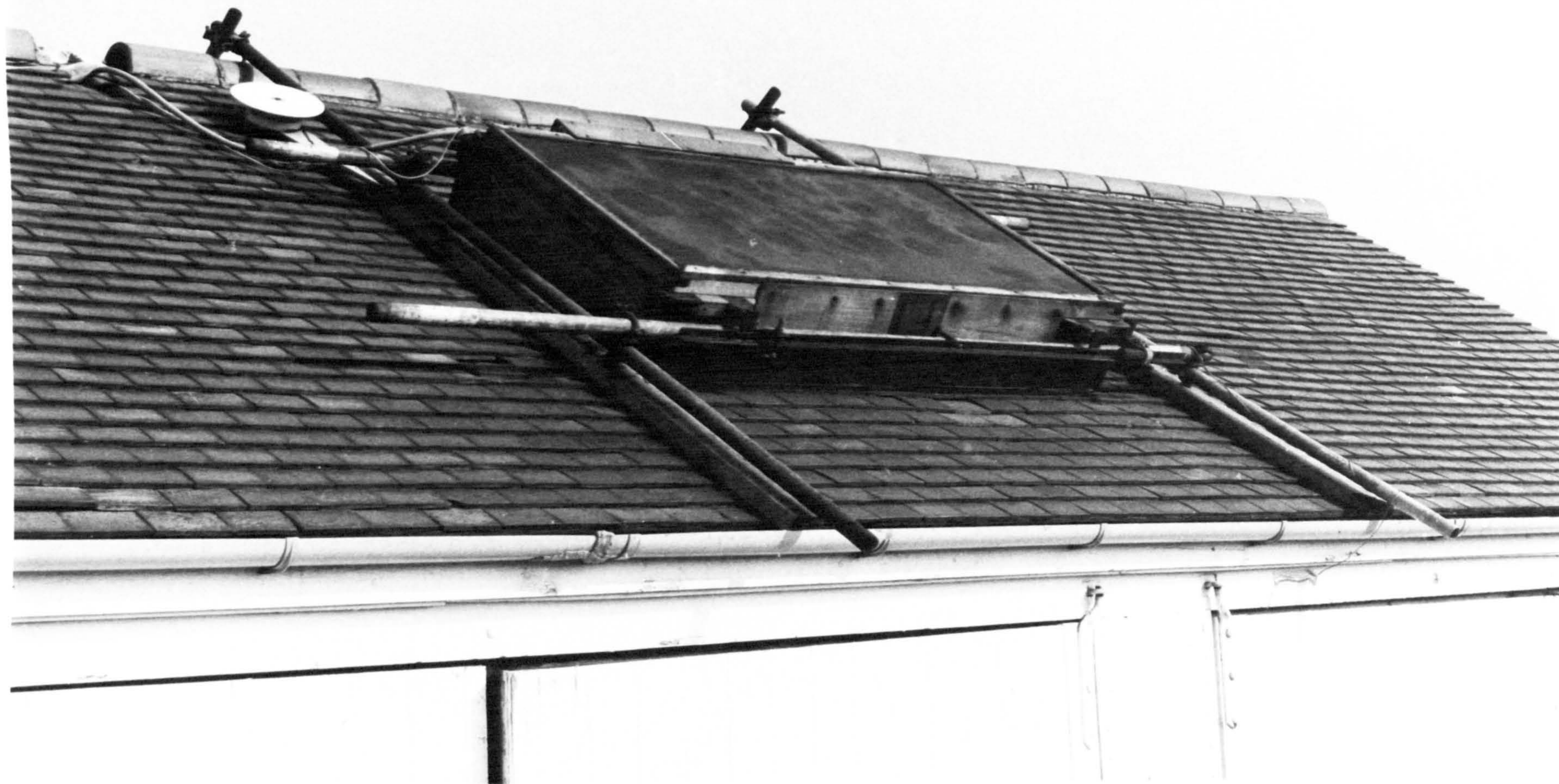
Figure 4.9 Close up view of heater plate assembly mounted on the test building roof
