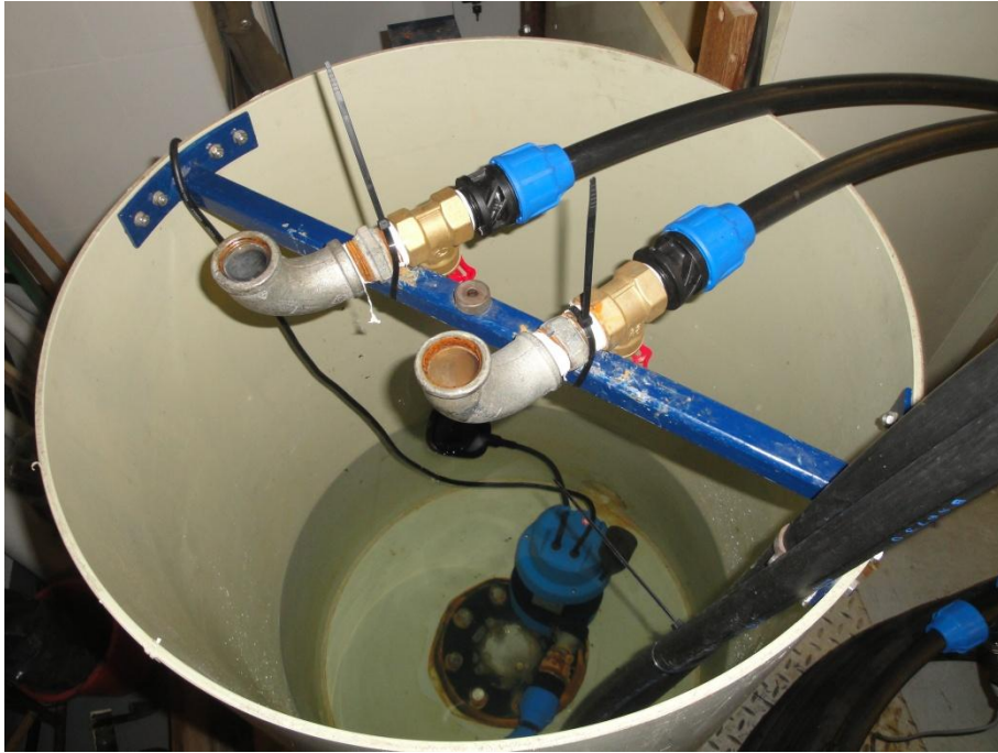
Figure 6-2 Collection reservoir with submersible pump showing pipe outlets with 90 bends to stop system drainage
