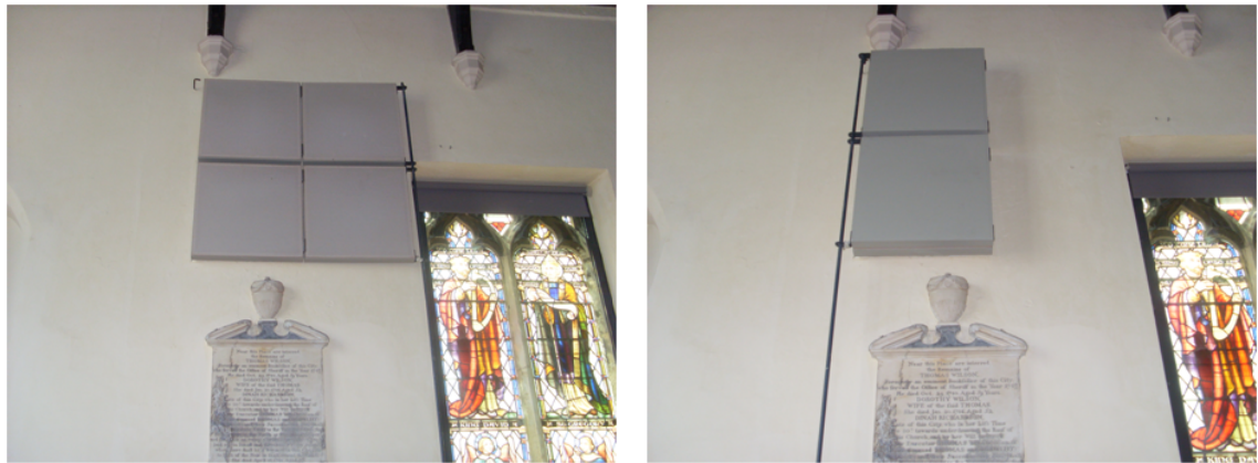
Figure 5.8 Acoustic panels set at the south wall. The 4 square absorbing panels (on the left) are folded in half, replaced by 2 reflecting panels (on the right).
