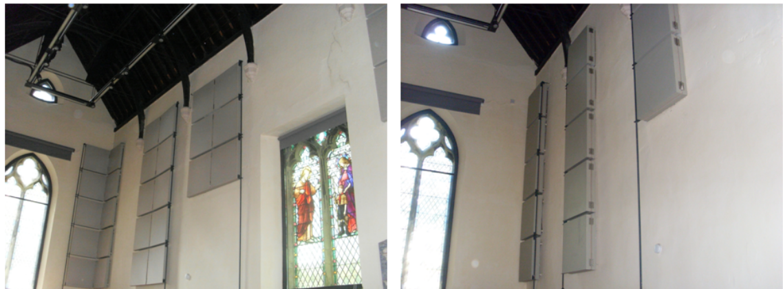
Figure 5.9 Acoustic panels set at the south-east walls. The 26 square absorbing panels (on the left) are folded in half, replaced by 13 reflecting panels (on the right).
