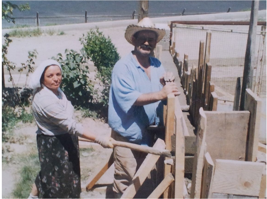
Photo 15-16: A Couple building a gecekondu in Ege/ Emine Öztürk's Family Photo Archive
