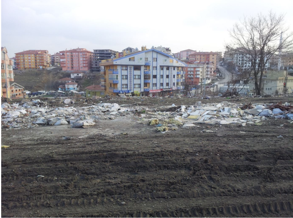
Photo 36: The gecekondus on the plots that are planned to be part of the main road were demolished.
