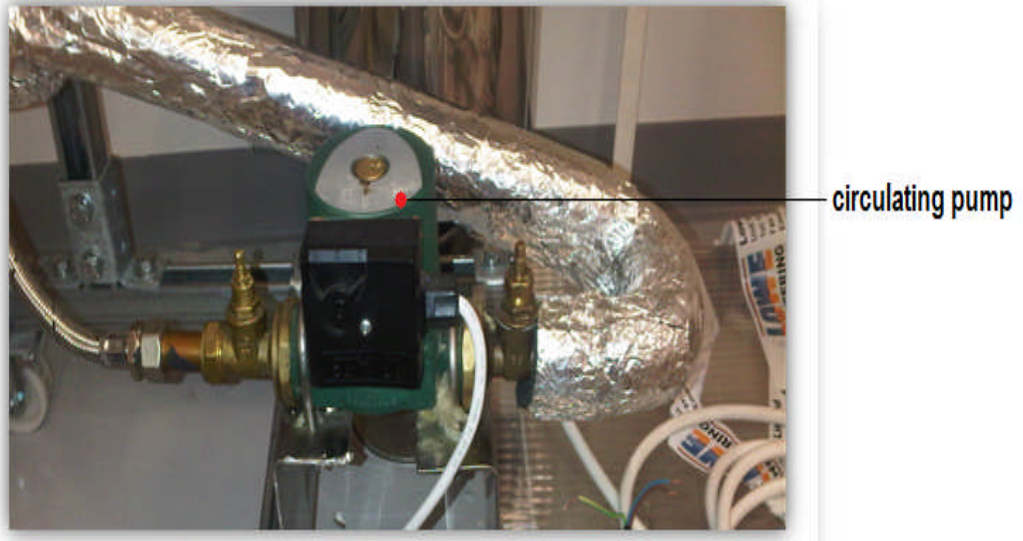
Figure 3-31: Photograph showing central heating pump used in the ESS Receiver Rig.
