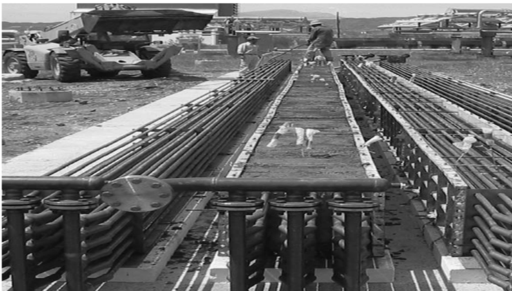
Figure 2-28: Solid media heat exchanger modules under construction for the WESPE project, Plataforma Solar de Almeria (PSA), Spain. (Source: [93] )
