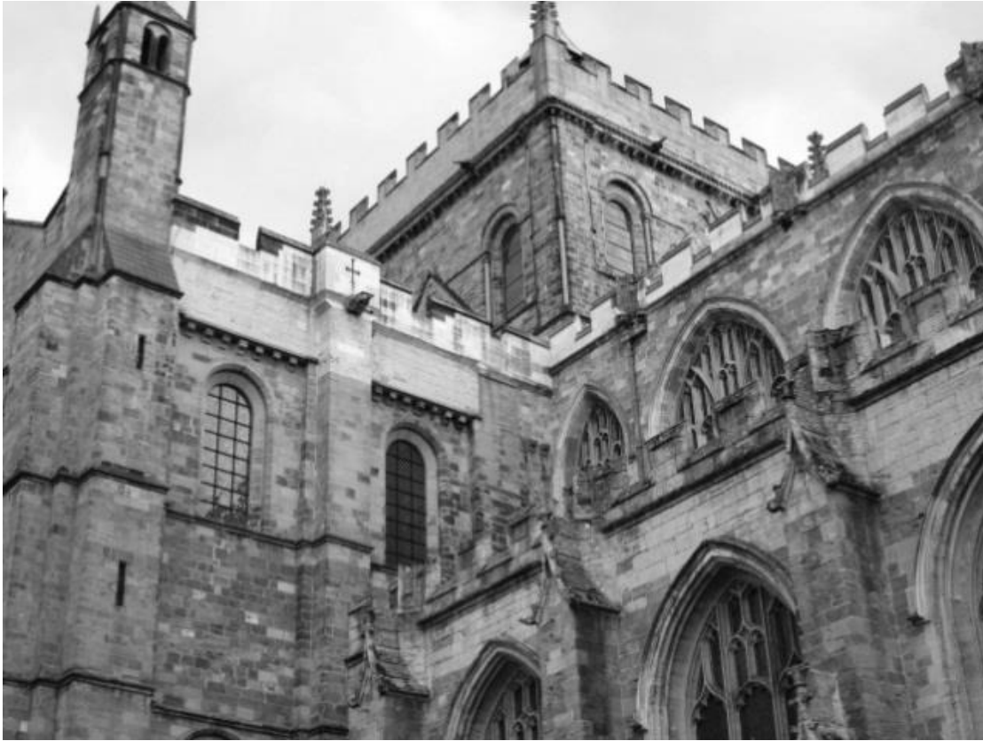
Figure 5.5: View of the tower from the northwest. This view shows the unaffected corner of the central tower. The lighter colour of the parapets of both the tower and the north transept arm indicate that they were constructed using magnesian limestone. The parapets on the eastern and western sides of the north transept were both raised as part of the c. 1465–1480 renovations (see Figure 5.4).
