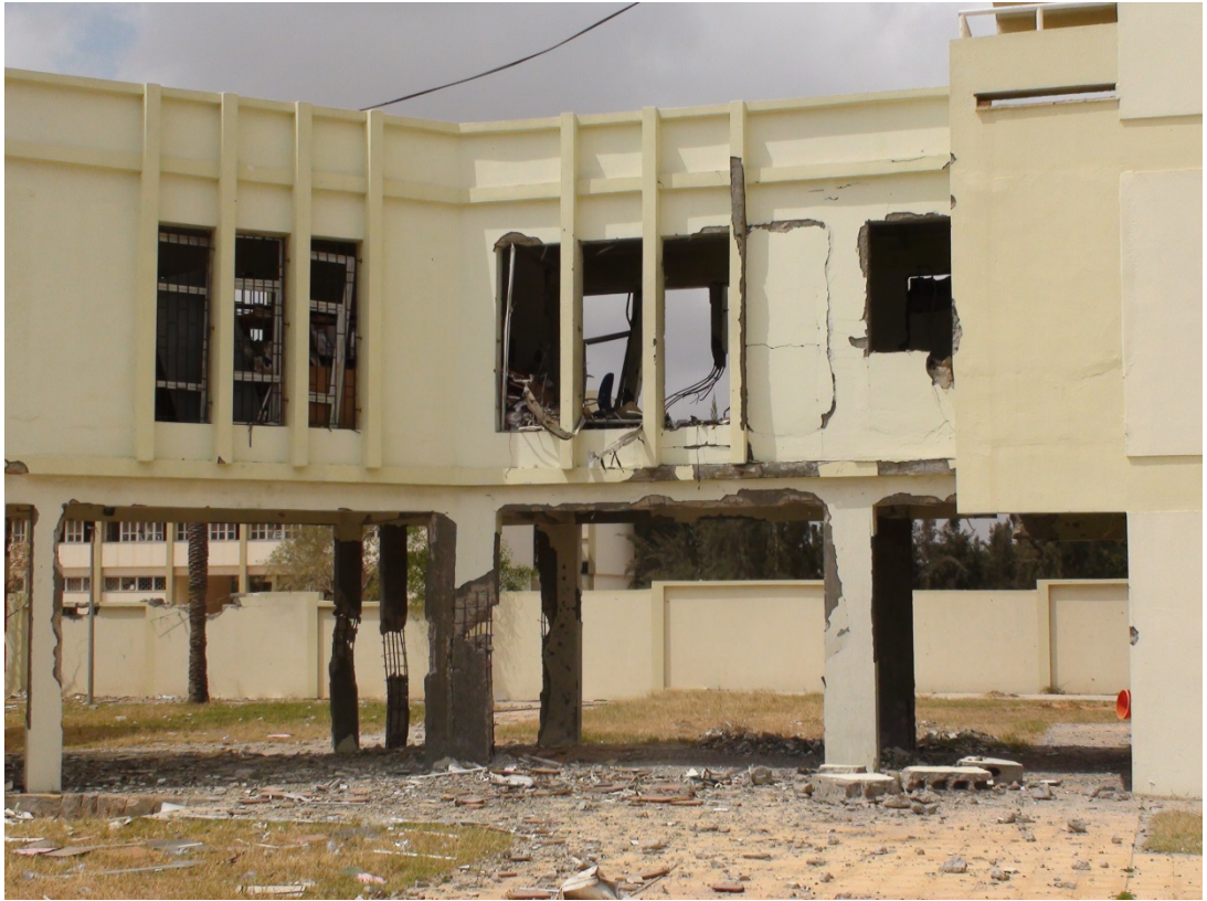
Photo D: Structural damage to Misrata University
