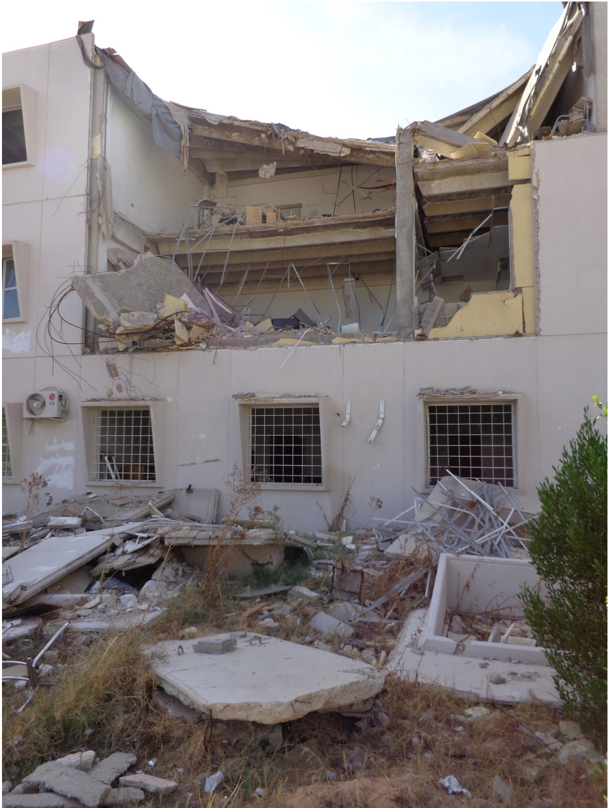
Photo C: Destroyed classroom at Tripoli University Campus B
