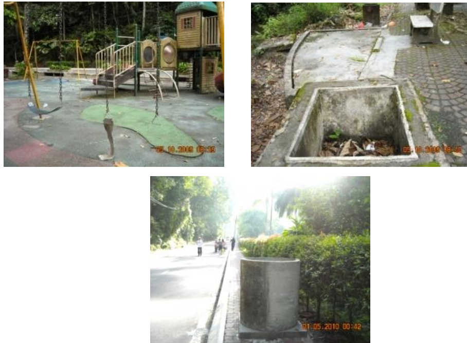
Figure 5.13 A few issues in Ampang Recreational Forest (Clockwise from top left: poor maintenance of play equipment for children, an uncovered manhole poses a danger to forest users, and a concrete rubbish bin located on a walkway)
