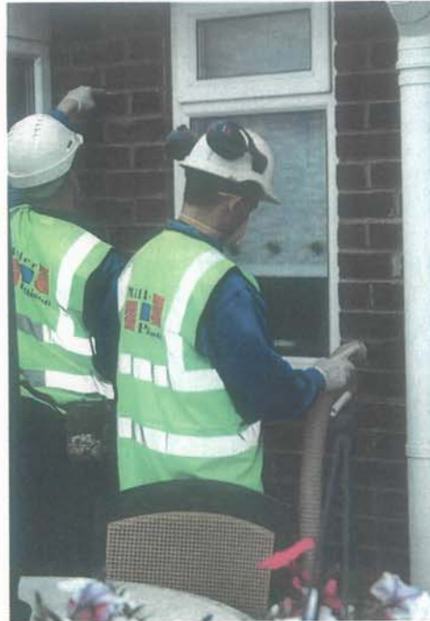
Loft and cavity wall insulation were energy conservation technologies offered for free under the Kirklees WarmZone programme. Photo: Yorkshire Energy Services
