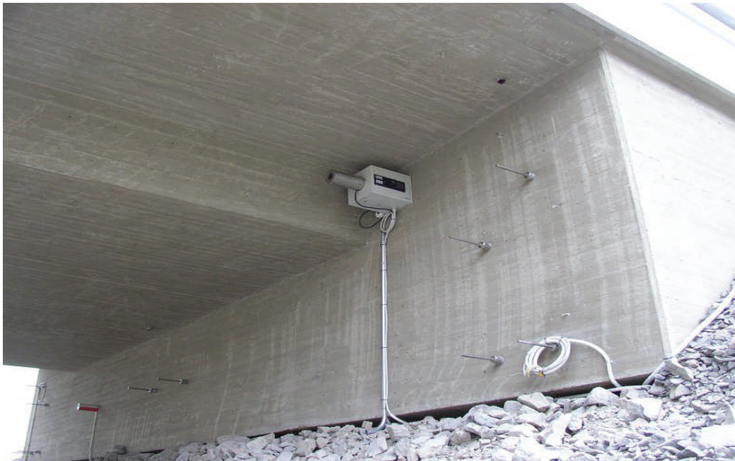
Figure 5.4: Bridge abutments showing laser distance-meter equipment and protruding end of steel bars (Kerokoski, 2006)
