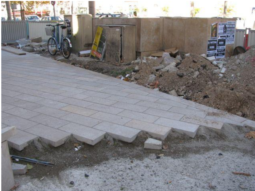
Figure 4.3: Flagstones being laid out in the Plan Cabanes, November 2010. Photograph: Roza Tchoukaleyska.
