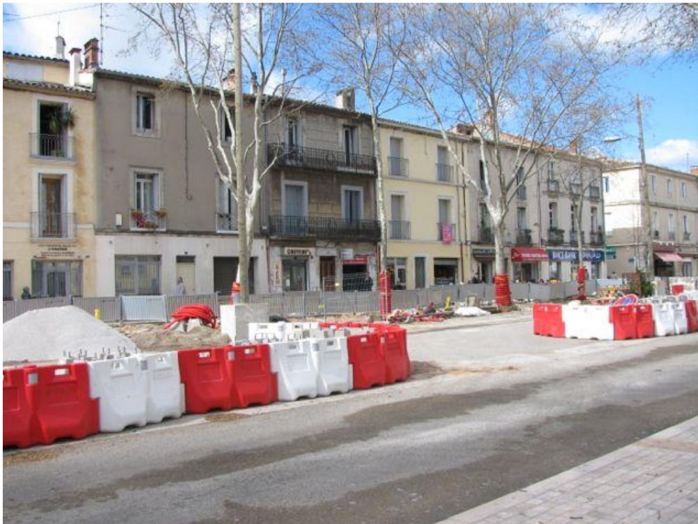
Figure 6.13: The Course Gambetta during tramway line #3 renovation, March 2010. Certain facades have already been renovated, others have yet to be started. Photograph: Roza Tchoukaleyska.
