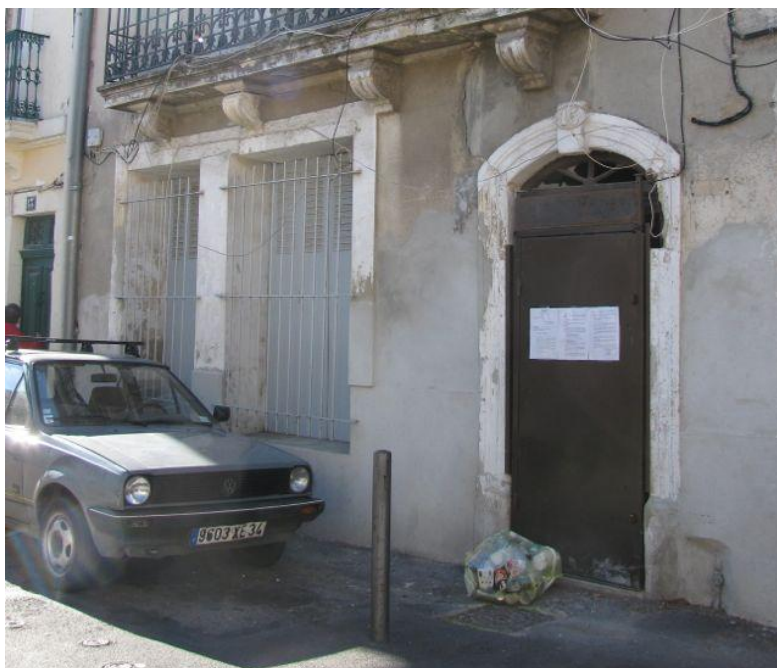
Figure 6.8: SERM / Grand Coeur renovation, 15 Rue du Père Fabre, with a brown metal SERM door on the building, November 2010. Photograph: Roza Tchoukaleyska.
