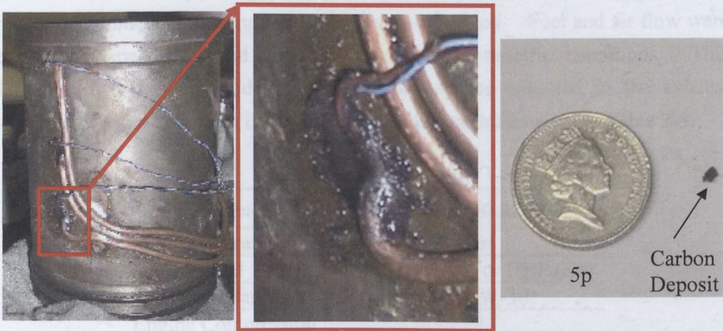
Figure 2-6 Photograph of TPS Liner, Sampling Pipe Attachment and Carbon Deposit
